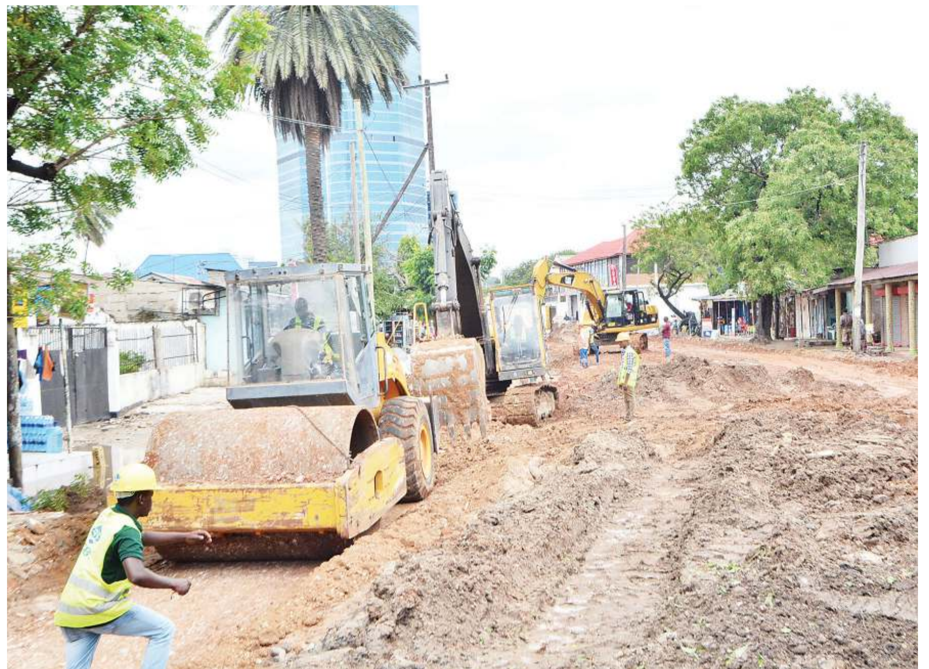
Igesa Street, which traverses Sinza Makaburini area in Dar es Salaam, undergoes rehabilitation yesterday. Photo: Correspondent Miraji Msala
