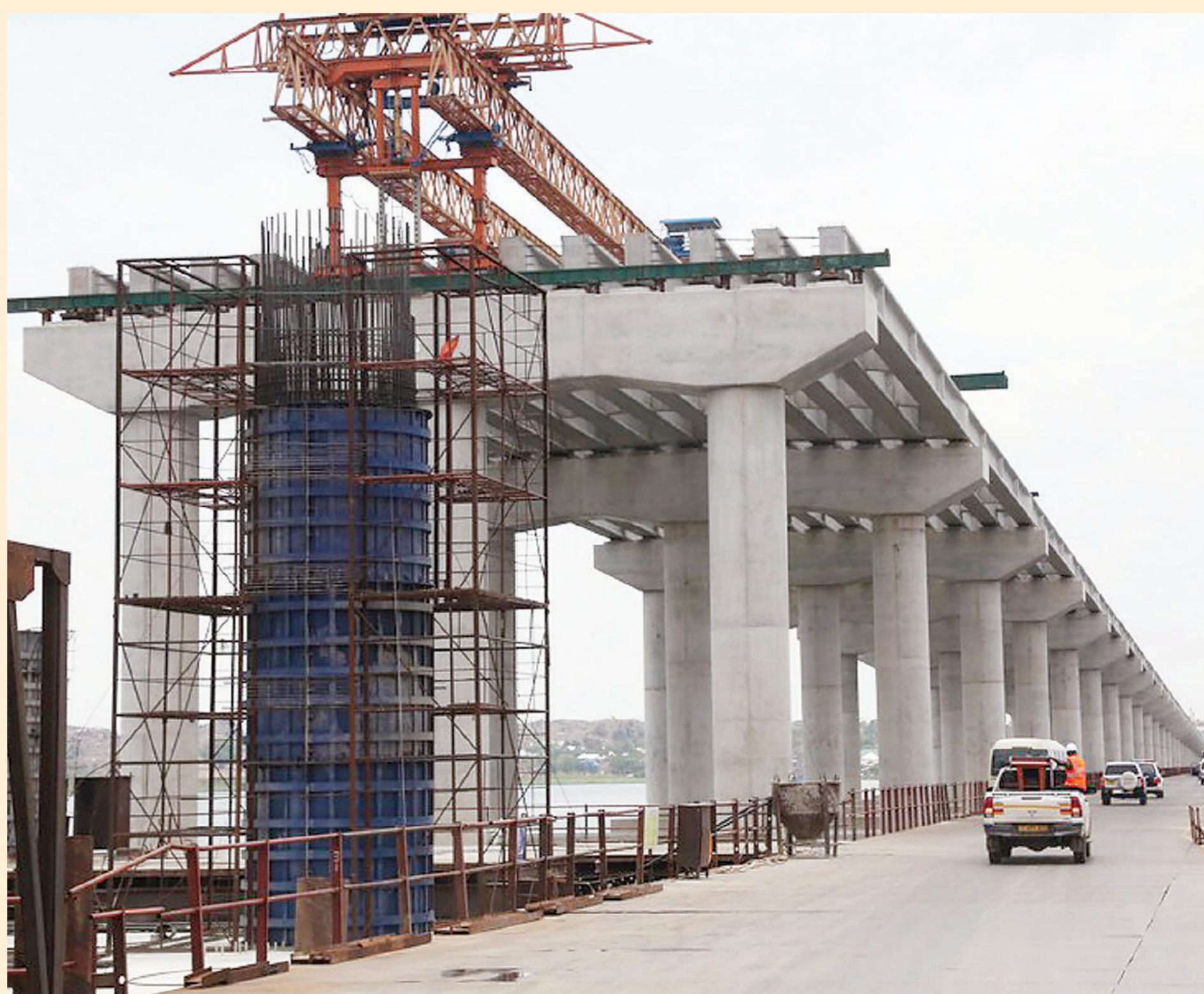
Construction site of the Magufuli Bridge project over Lake Victoria in Mwanza Region. Some Tanzanian MPs said that projects being undertaken under the Belt and Road Initiative (BRI) framework are helping the East African nation to open up its economy.
