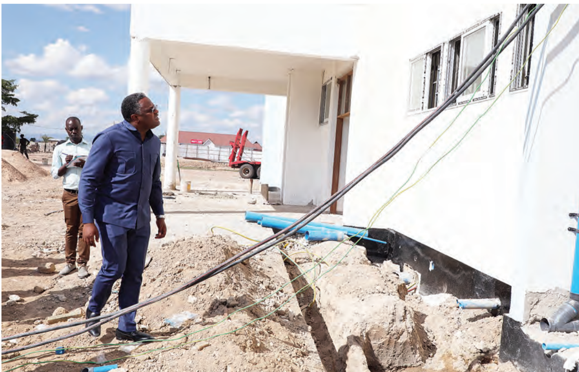
Dr Jim Yonazi, Deputy Permanent Secretary in the Communications and Information Technology ministry, inspects national fibre network at Uhuru Hospital in Chamwino District on Thursday. Photo: Guardian Correspondent
