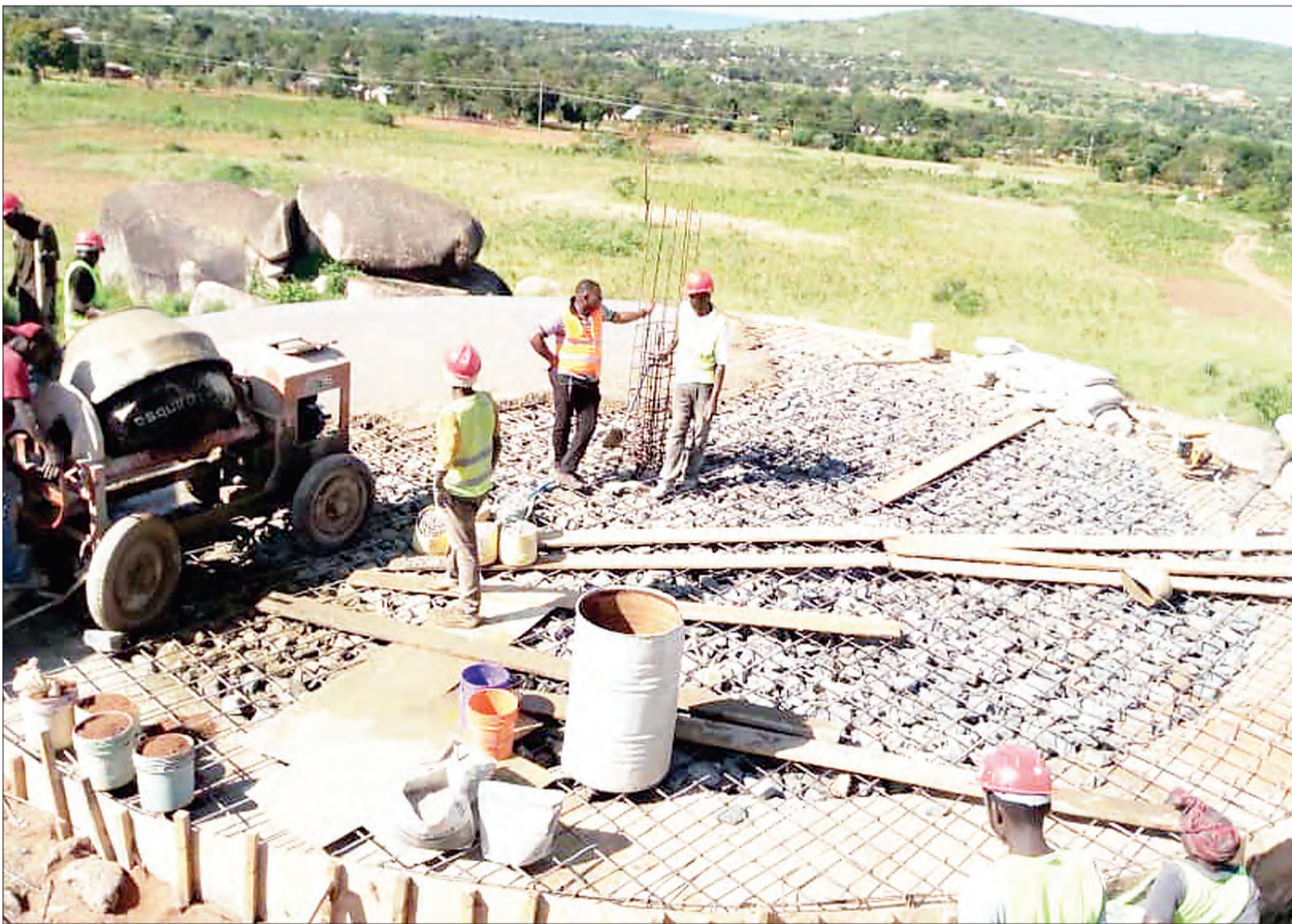
Rural Water Supply and Sanitation Agency technicians busy with the construction of a 300,000-litre water tank at Nyakatende in Musoma District on Thursday. Photo: Guardian Correspondent
