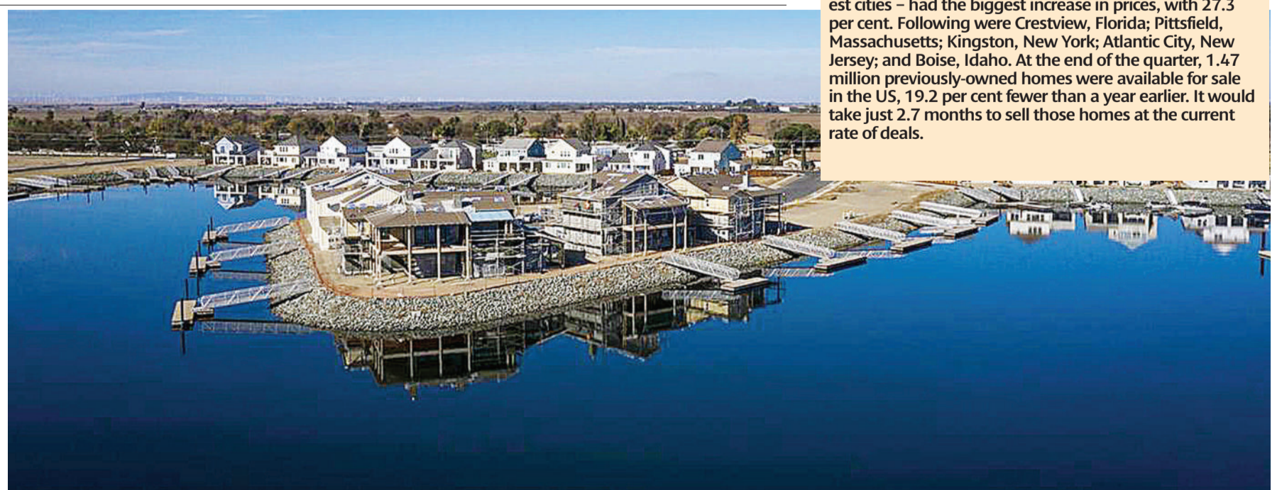
The Delta Coves housing development under construction on Bethel Island, California. Prices for single family homes jumped 12% across the US in the third quarter, according to new statistics.
