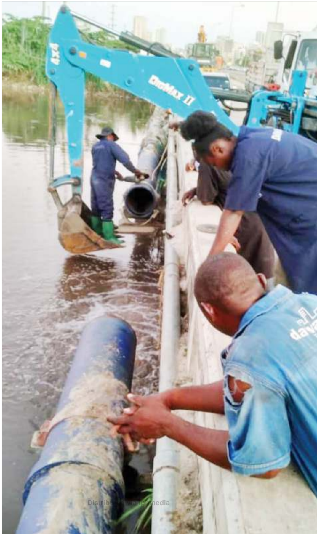
Dar es Salaam Water and Sanitation Authority technicians repair a pipe at Jangwani in the city, giving residents of parts of Ilala municipality hope of the resumption of normal supply of the precious liquid soon. Photo: Guardian Correspondent
