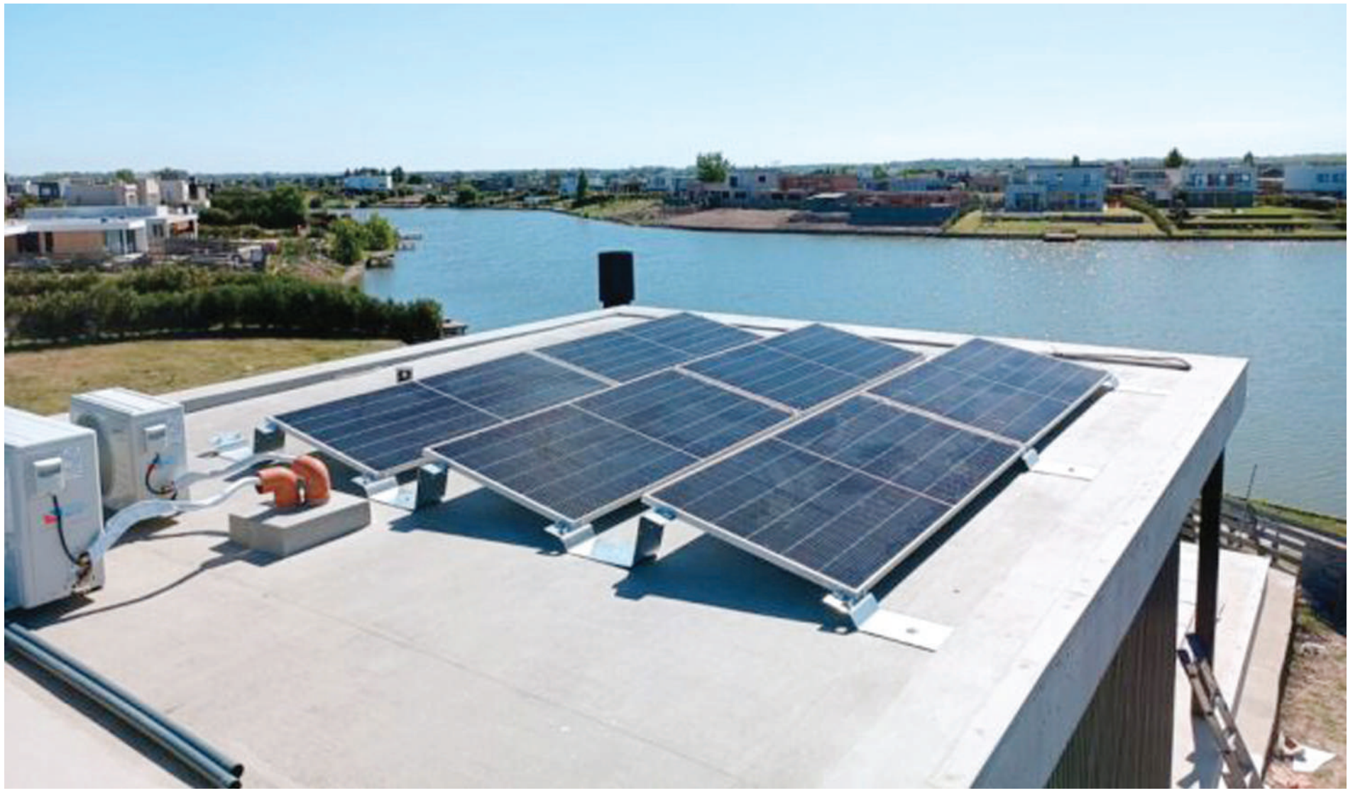
Aerial view of the 5000 square meter roof full of solar panels, in one of the pavilions of La Rural, the busiest fair and exhibition center in Buenos Aires. It is the largest private solar park in the capital of Argentina and required an investment of almost one million dollars. CREDIT: Courtesy of La Rural
