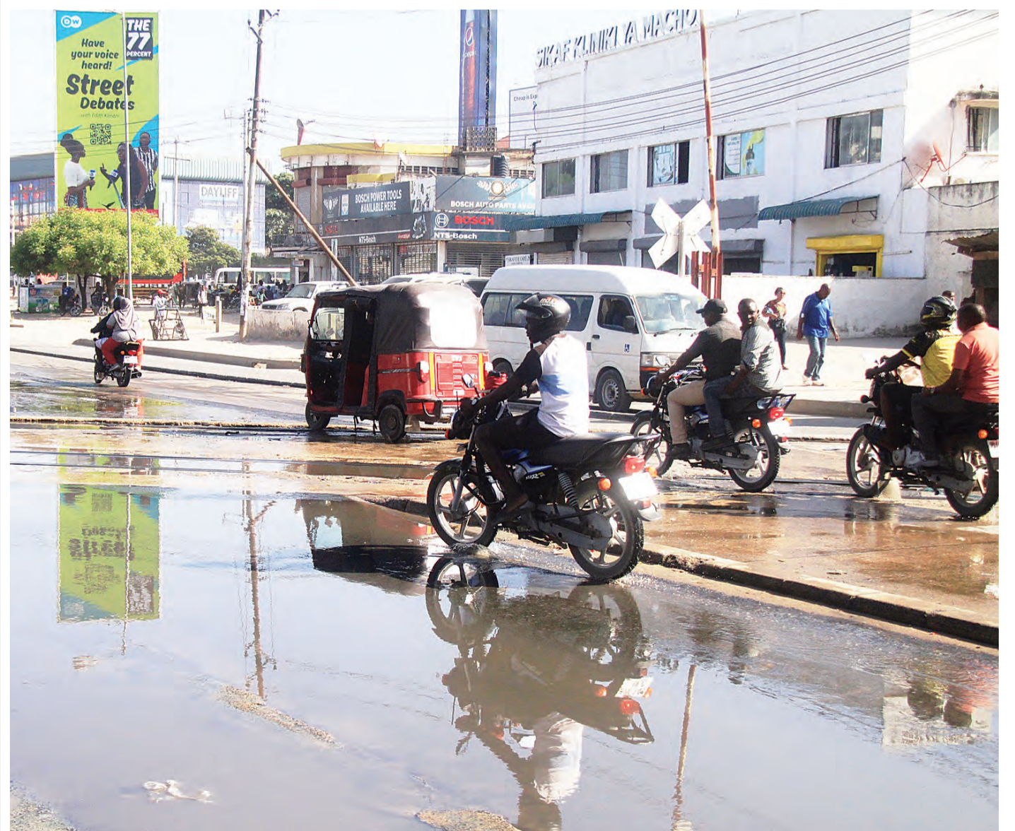
What appears to be "water" covering a section of a road has completely nothing to do with rain but is, in fact, stinking sewage from a drainage chamber near the Kamata section of Dar es Salaam's Nyerere Road - as found yesterday. Photo: Correspondent Jumanne Juma
