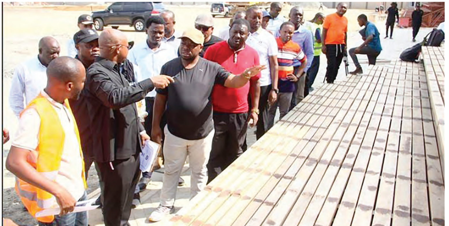
Dar es Salaam Regional Commissioner Albert Chalamila (front in black t-shirt) inspects the construction of the Kinondoni Municipal Council (KMC) stadium at Mwenge in Dar es Salaam over the weekend. PHOTO: JUMANNE JUMA
