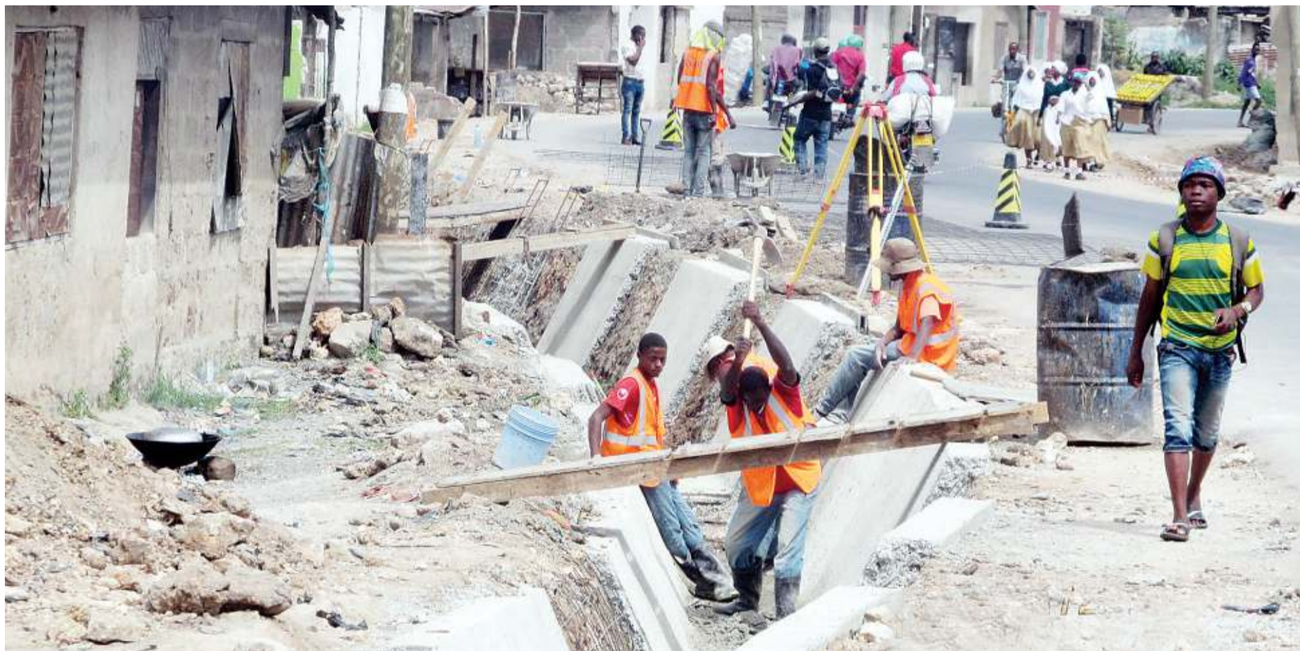
Work in progress on a trench at a section of a road being built to link Dar es Salaam's Mwananyamala and Tandale suburbs, as found yesterday. Photo: Correspondent Sabato Kasika
