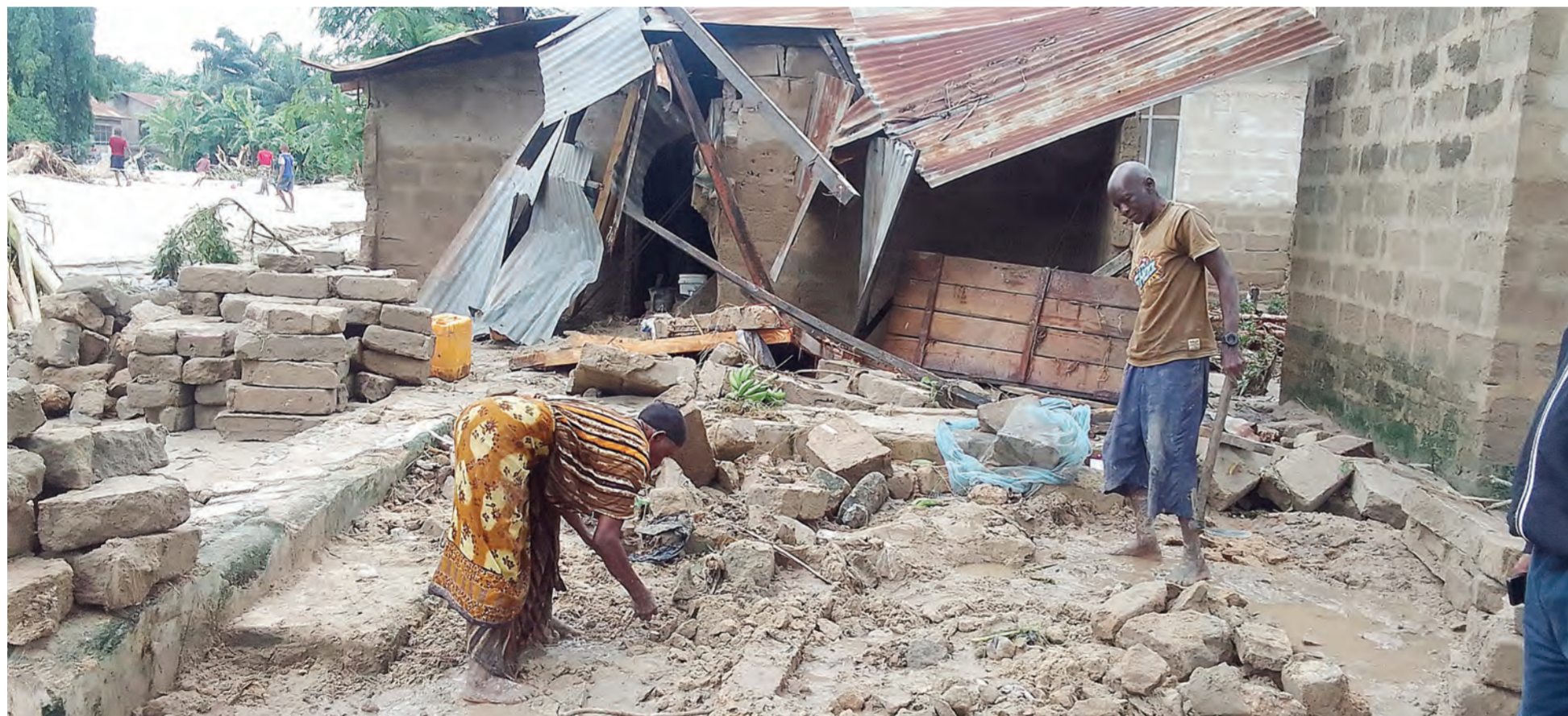
PICKING UP THE PIECES: Residents of Dar es Salaam's Tegeta Machinjioni suburb collect bricks yesterday after hours of incessant heavy rain demolished their house at the weekend. Photo: Correspondent Elizabeth Zaya
