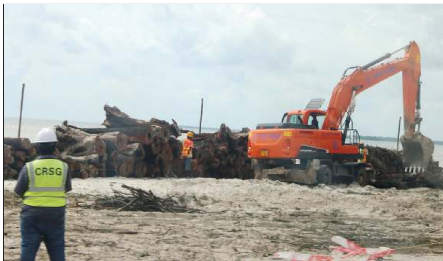
An excavator deployed by China Railway Seventh Group at work at the starting point of the construction of Dar es Salaam's 6.23-km Selander Bridge, which is expected to run from near Aga Khan Hospital - over Indian Ocean waters - right to Coco Beach. Implementation of the 556.1bn/- project is lined up to take 36 months, with the Tanzanian government contributing 49.457bn/- Photo: Selemani Mpochi.
