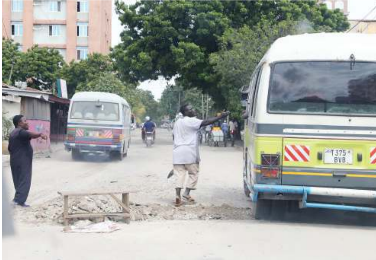
A resident of Lindi Street in Ilala municipality, Dar es Salaam, demands money from a commuter bus conductor yesterday as contribution to self-help efforts to repair a road damaged by rain. Photo: Selemani Mpochi
