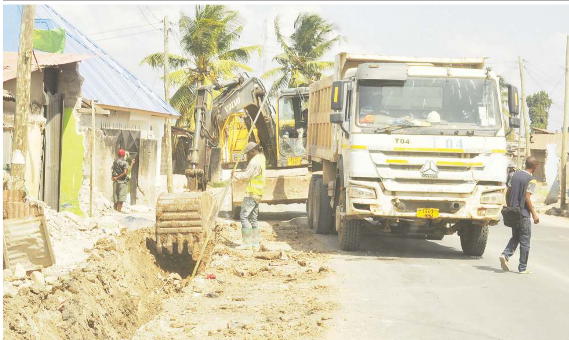
Construction of a tarmac road linking Mwananyamala kwa Manjunju and Tandale kwa Mtogole suburbs in Dar es Salaam's Kinondoni Municipality in progress, as found yesterday. Photo: John Badi
