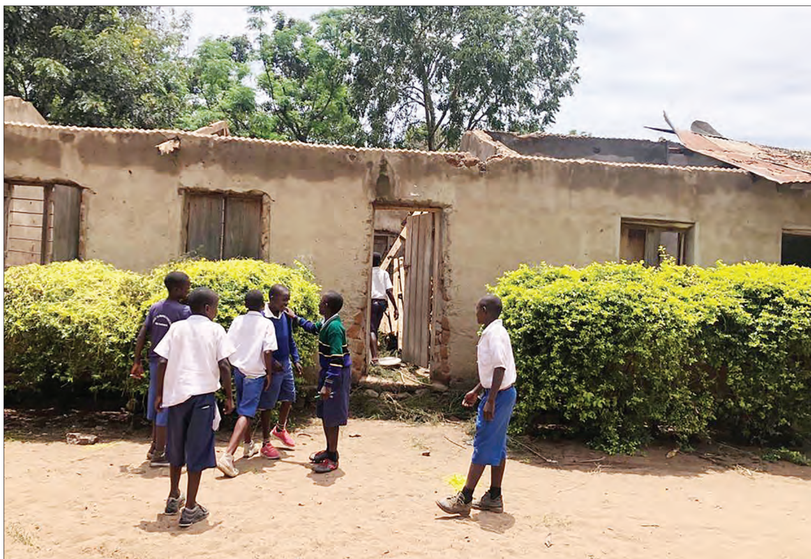
Lyaseembe Primary School pupils at Murangi ward in Musoma District, Mara Region standing outside their classroom yesterday whose roof was damaged during heavy rains over the weekend. Photo: Correspondent
