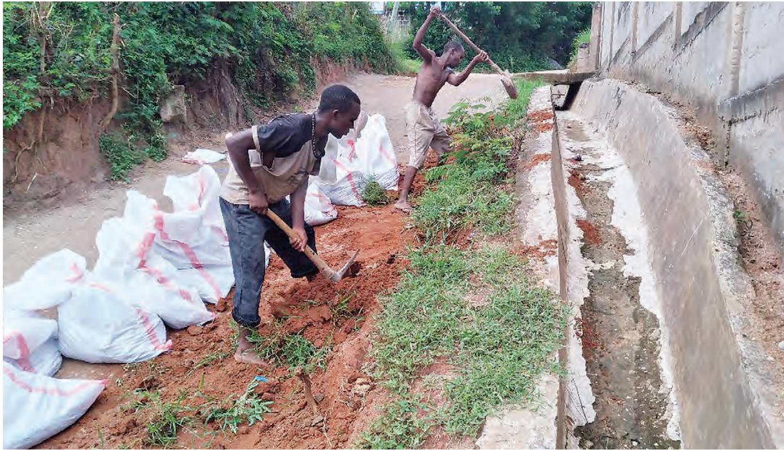
Preparations under way for the rehabilitation of a road at Tabata-Kisukuru Ephata in Dar es Salaam yesterday. Photo: Correspondent Joseph Mwenda-pole
