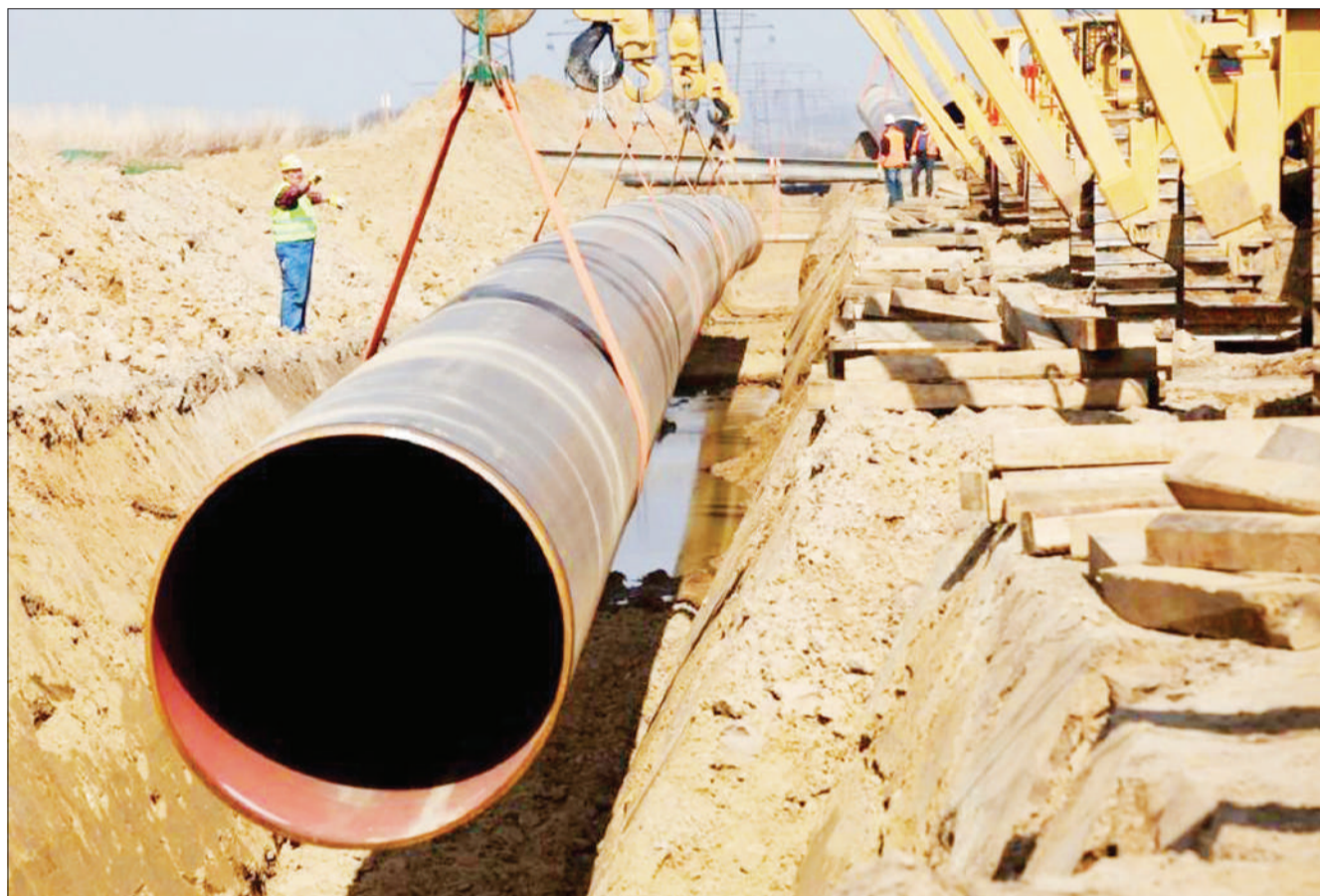
A scene from one of the sites of the laying of the 1,445-km East African Crude Oil Pipeline to run from Hoima in Uganda to Tanga Port in Tanzania, with implementation of the mega-project expected yet to start in earnest. File Photo
