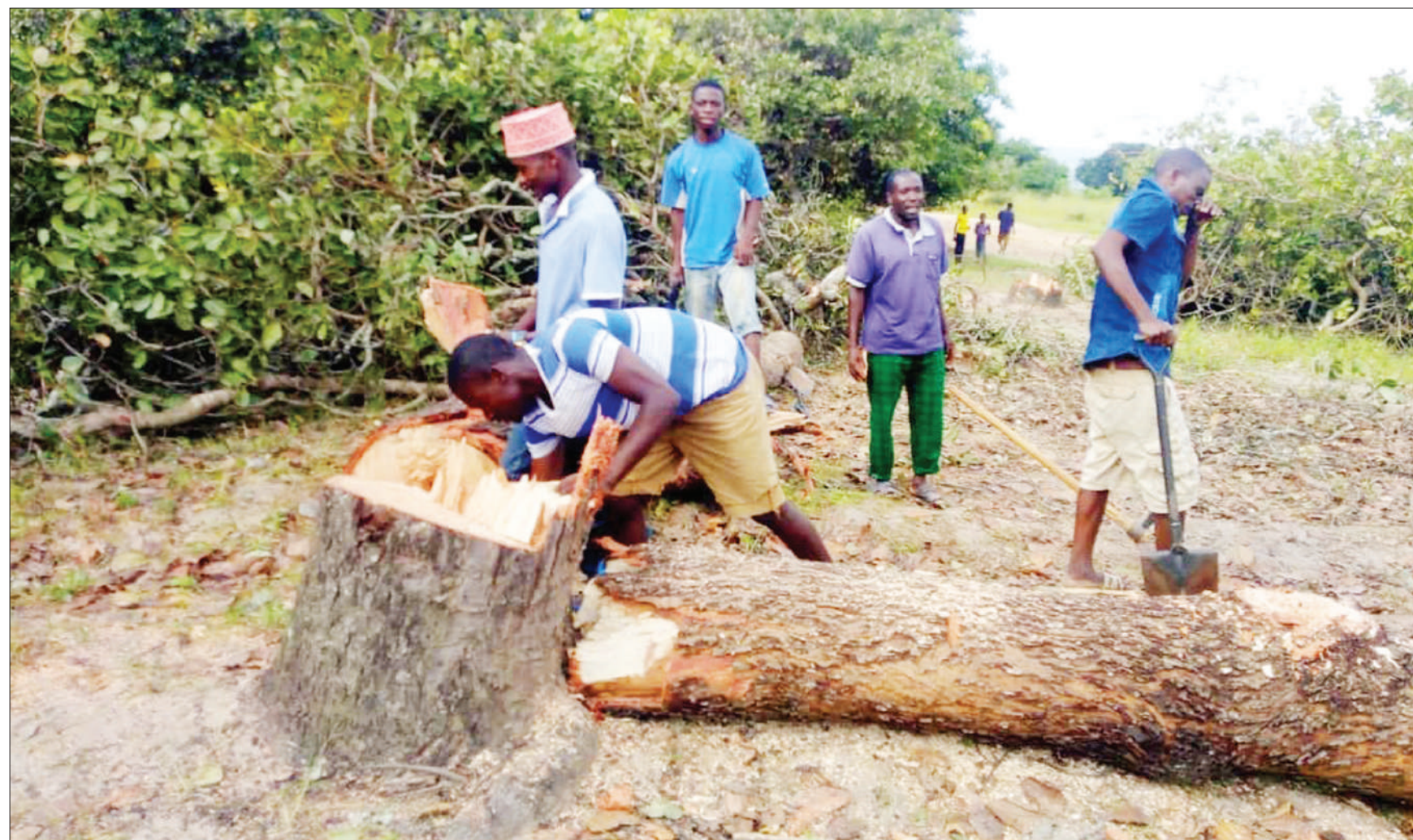
Residents of Kajima in Tunduru District move to clear a 16-km stretch of bush earlier this week to pave the way for the construction of a road to neighbouring Matemanga and "woo" vehicle owners into making it to their village. Photo: Correspondent Steve Chindiye
