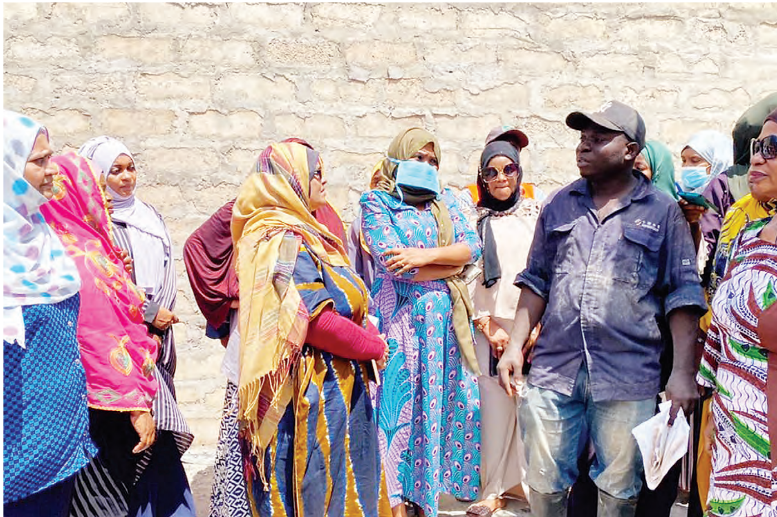
The foreman (in cap) overseeing the construction of the proposed Gender Centre of the Zanzibar chapter of the Tanzania Media Women's Association (Tamwa) briefs the association's members at the site of the project – at Tunguu – at the weekend. Photo: Rahma Suleiman
