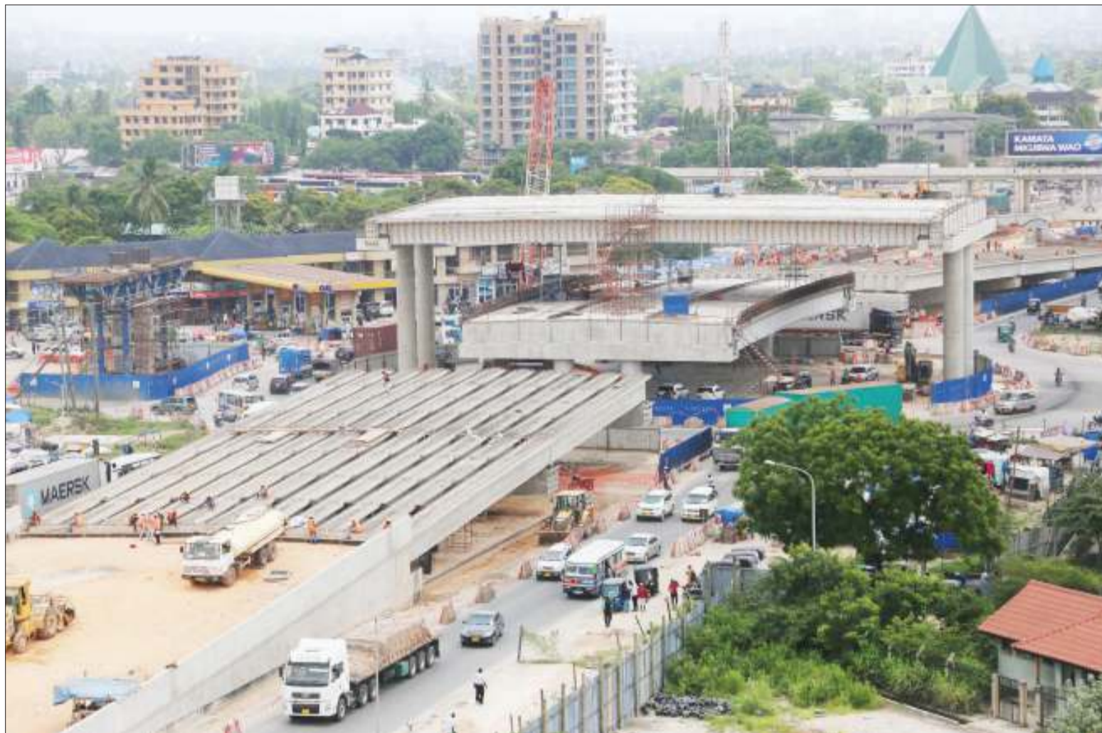
The construction of Dar es Salaam's Ubungo interchange at the Morogoro Road/Mandela Road/Sam Nujoma Road intersection by the China Civil Engineering Construction Corporation is registering steady progress. Chief Photographer Selemani Mpochi captured this scene yesterday
