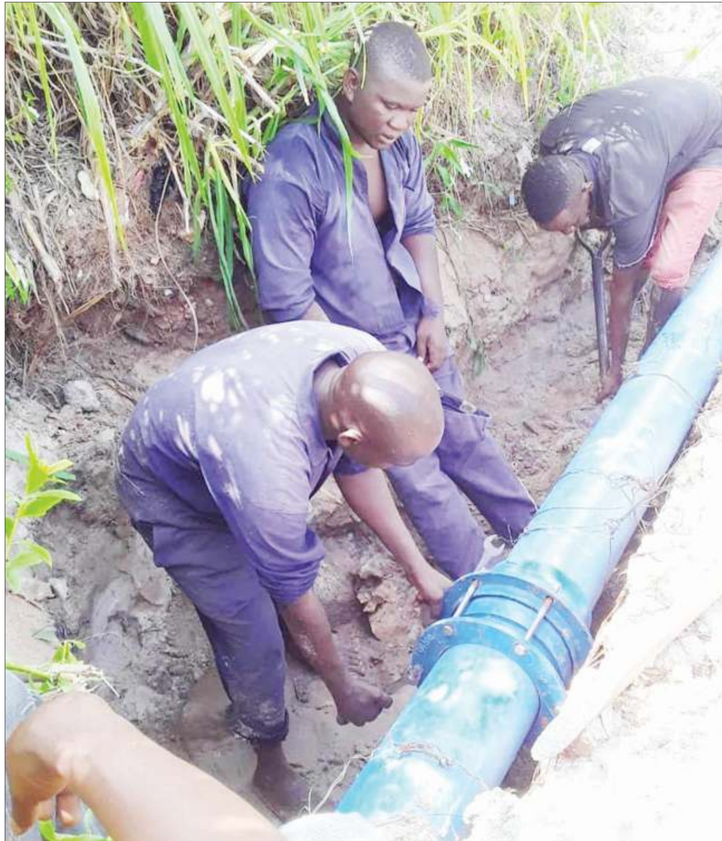
Dar es Salaam Water and Sanitation Authority (Dawasa) technicians repair a water pipe at Bonyokwa in Ubungo District yesterday. Photo: Guardian Correspondent
