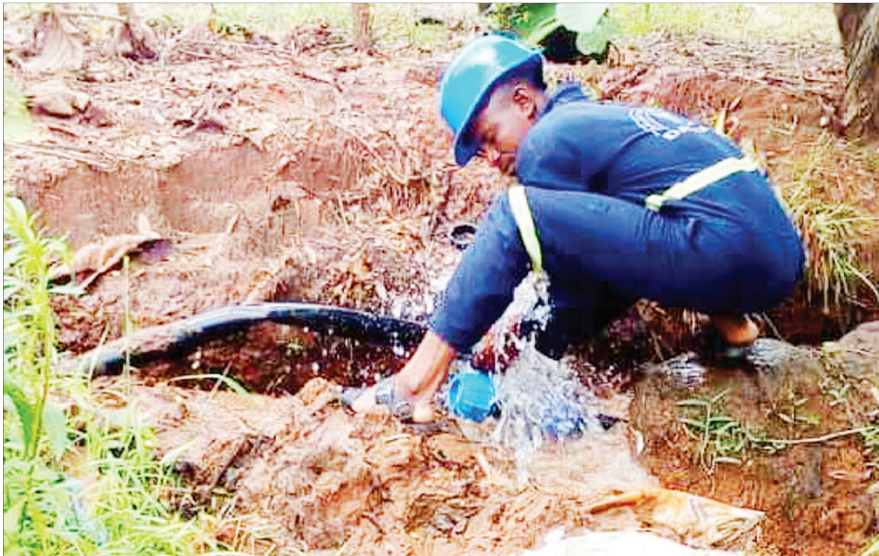
Adam Shamte, a technician with the Dar es Salaam Water and Sanitation Authority's Tegeta station, fixes a leaking pipe in the city's Salasala suburb yesterday. Photo: Guardian Correspondent
