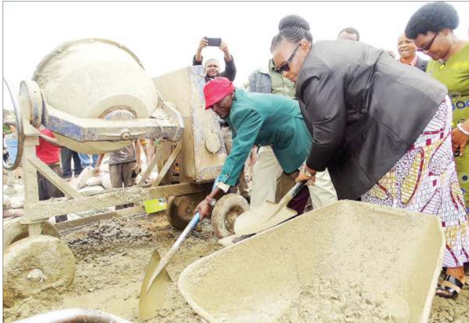
Karatu district commissioner Theresia Mahongo (R, foreground) helps in laying the foundation stone for boys' dormitories at Kilimamoja Secondary School, which is being developed into a boarding institution. Photo: Guardian Correspondent
