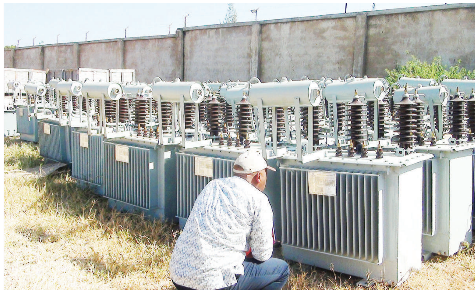
Rural Electrification Agency board member Henry Mwimbe pictured at the weekend inspecting a transformer awaiting installation at the site of a project in Singida Region. Photo: Correspondent Jumbe Ismail
