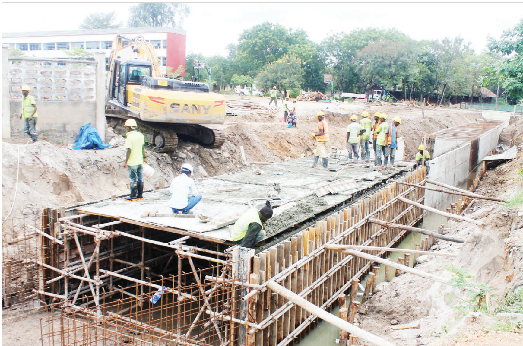
Construction of a sewage system in progress beside Dar es Salaam's Chang'ombe Road yesterday under the oversight of China Railway Group contractors. Photo: Correspondent Jumanne Juma
