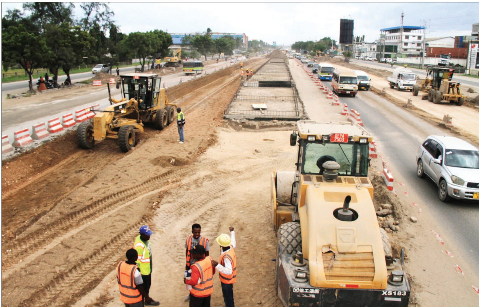
An aerial view of progress in the implementation of the Dar es Salaam rapid transit bus road project, as captured yesterday on a section of the Vingunguti-Gongo la Mboto stretch of Nyerere Road. Photo: Correspondent Jumanne Juma
