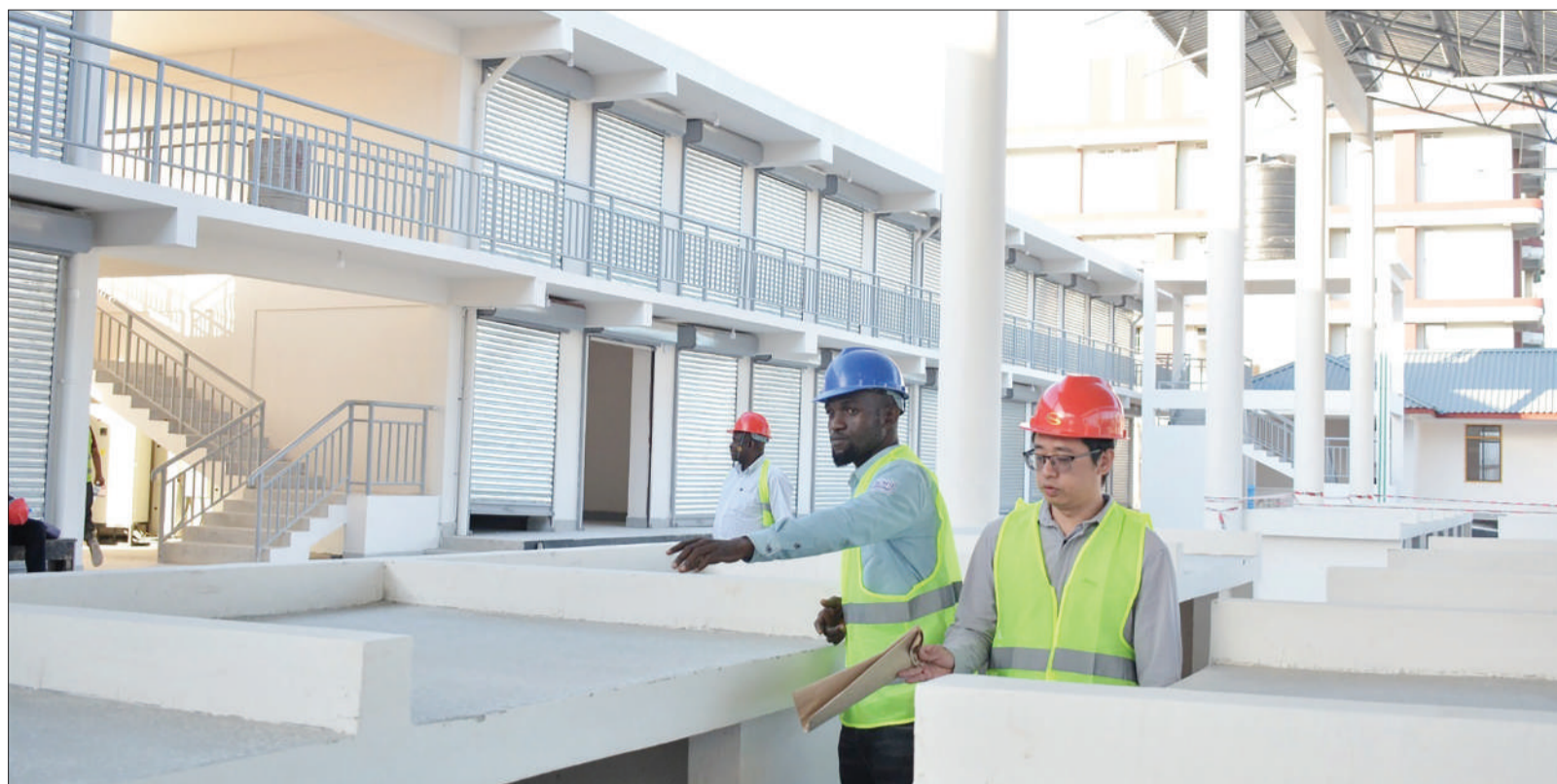
Hans Charles (in blue helmet), construction supervisor of Dar es Salaam's Mbagala Zakhem Market, briefs Group Six International Ltd project manager Liu Jianhua (R) yesterday before handing over to Temeke municipality the now-completed 2.4bn/- facility put up under Dar es Salaam Metropolitan Development Project. Photo: Guardian Correspondent
