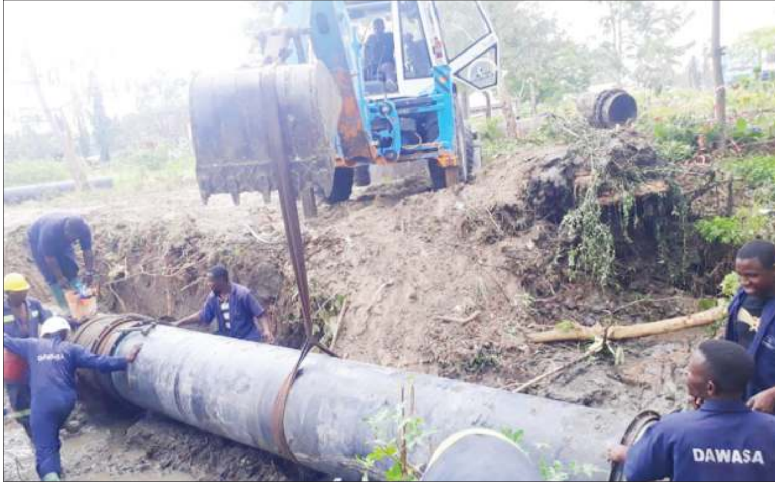
Dar es Salaam Water and Sewerage Authority (DAWASA) technicians replacing a dilapidated water pipe at Kibaha Maili Moja in Coat region yesterday. The replacement of old water pipes is one of the strategies to improve service. Photo: Correspondent Frank Monyo
