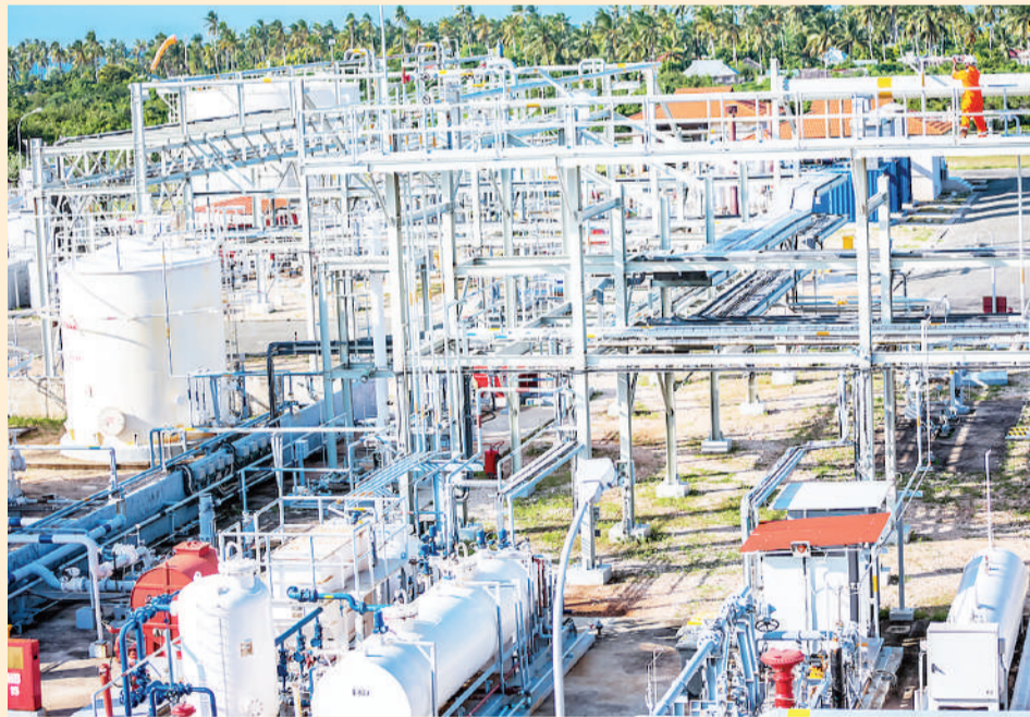
Songo Songo natural gas plant
