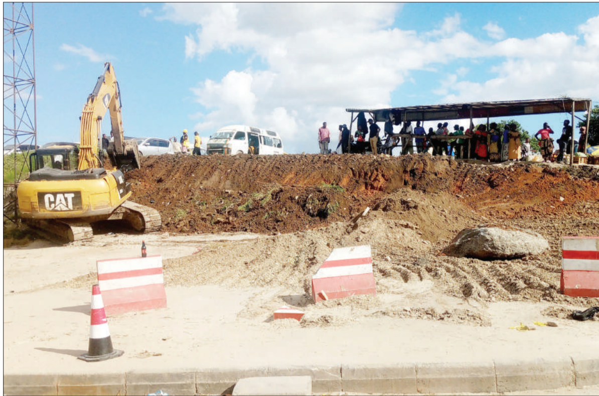
Expansion of the Dar es Salaam-Kibaha stretch of the Morogoro highway well in progress at the commercial city's Kimara Mwisho section on Monday, effectively ending all dreams of staying put in the area with whatever business they had been doing there. Photo: Correspondent Sabato Kasika
