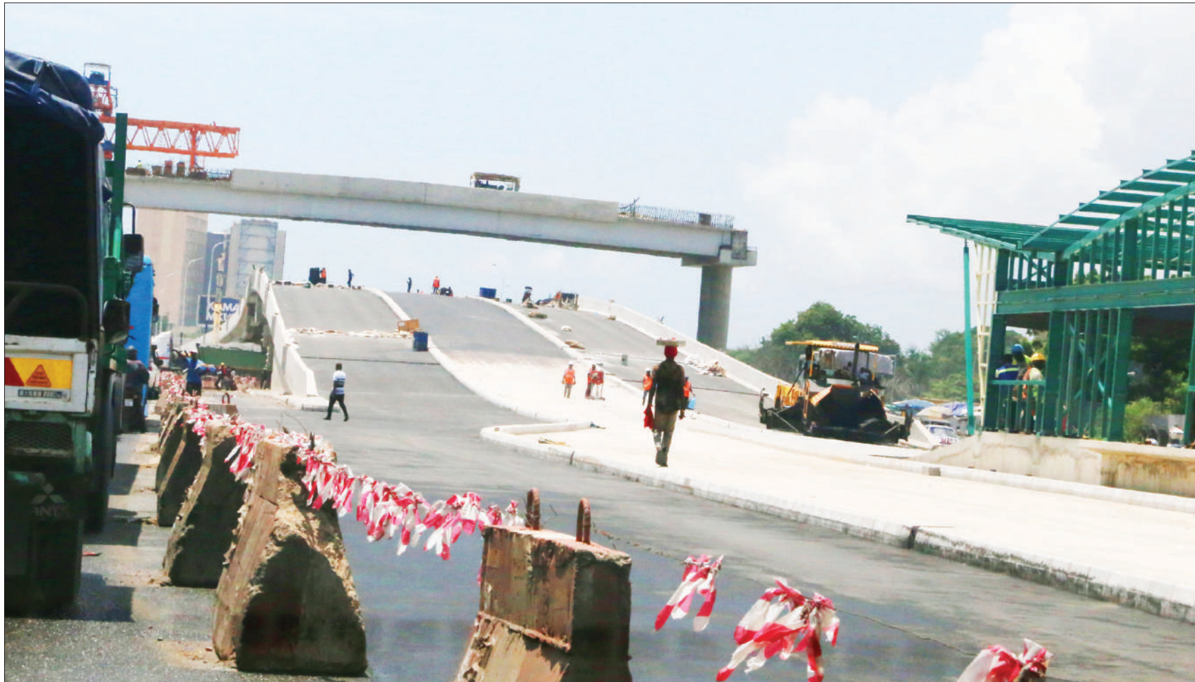
This is a section of the Ubungo interchange at the Morogoro Road/Mandela Road intersection in Dar es Salaam, as captured yesterday. The facility is still undergoing construction. Photo: Selemani Mpochi
