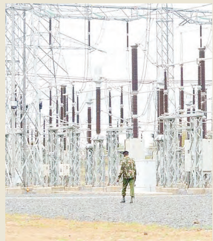
A police officer patrols substation of Kenya Electricity Transmission Company Limited in Suswa
