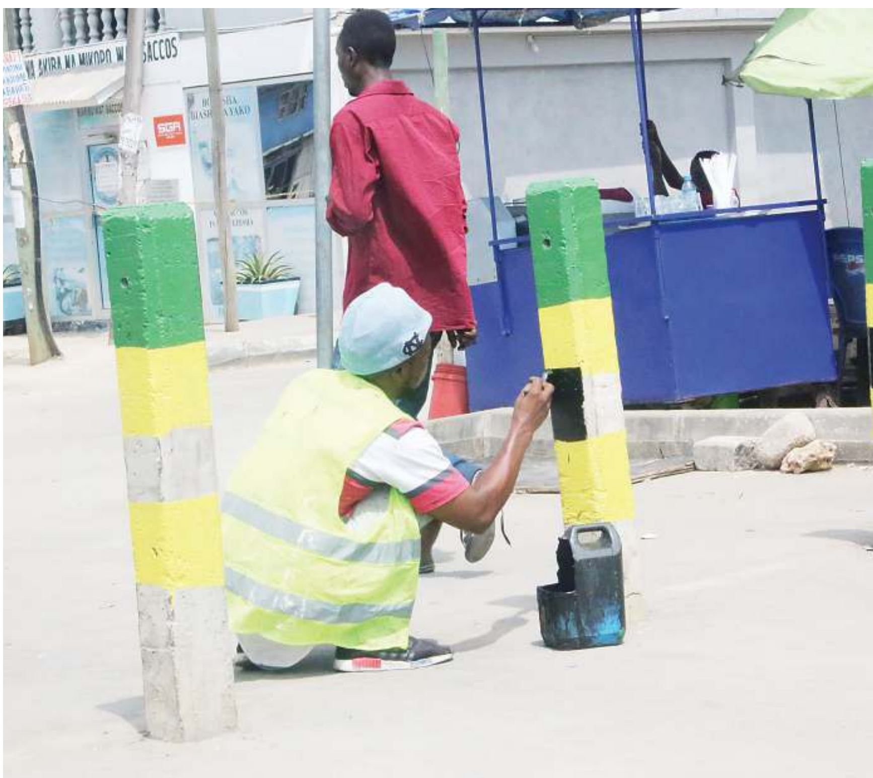
Concrete poles along the pavement of Dar es Salaam's Kawawa Road undergo painting as part of effort to add a touch of beauty to the city, as found yesterday. Photo: Selemani Mpochi
