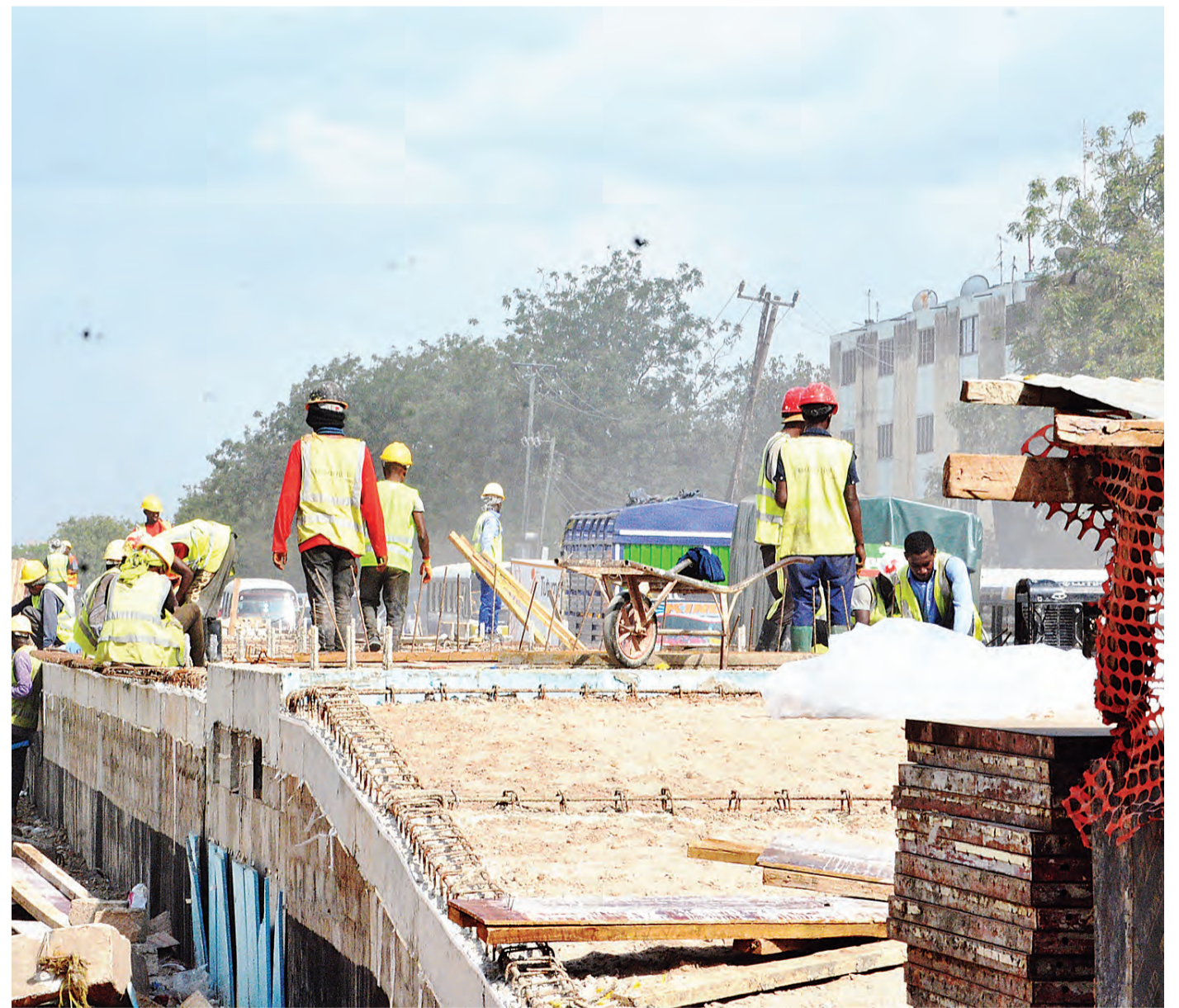
Construction of flyover in progress yesterday at a section of the Ilala stretch of Dar es Salaam's Kawawa Road. Photo: Correspondent Miraji Msala
