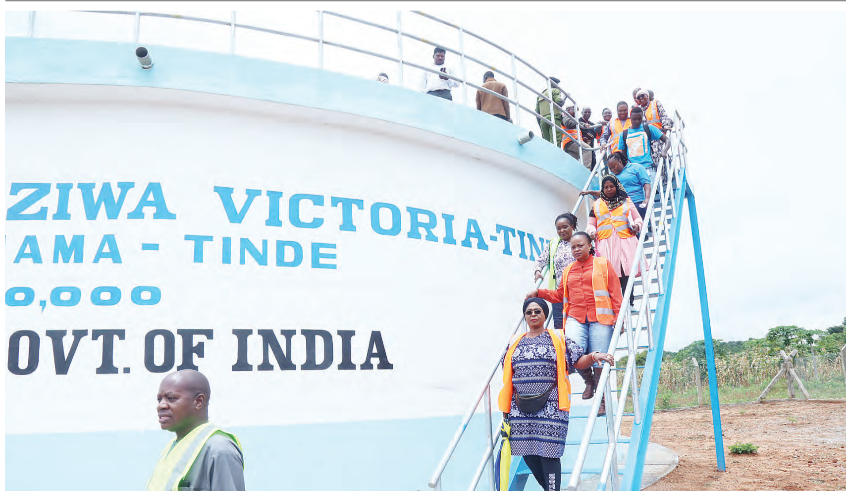
Jackson Kiswaga (L), Chairman of the Parliamentary Water and Environment Committee, pictured at Buchama in Tinde ward, Shinyanga District, on Thursday leading members of the committee on an inspection tour of a 1.15 million-litre Lake Victoria water tank project at Tinde-Shelui whose implementation cost 24.47bn/-.
