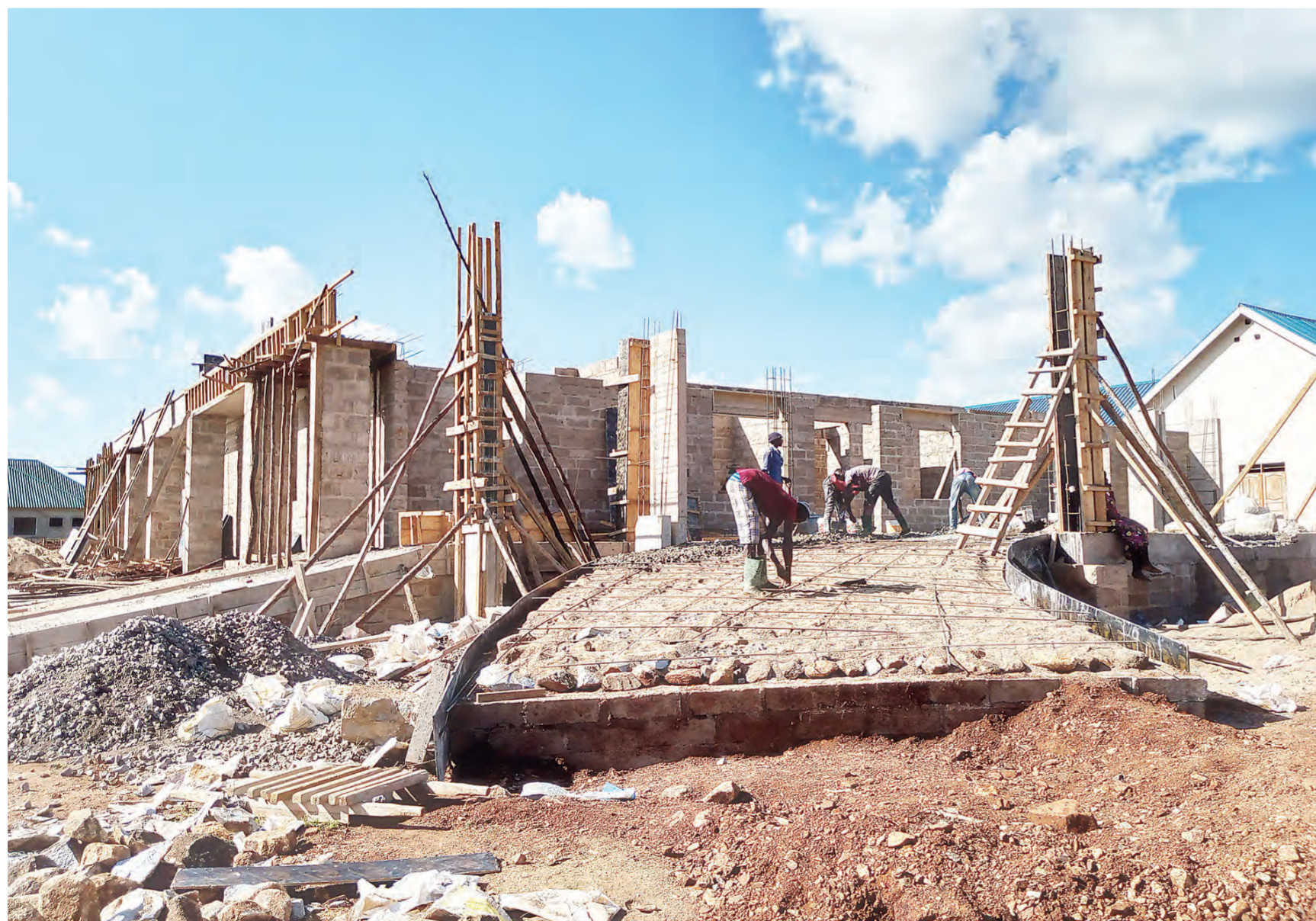
Construction of a new government hospital for Musoma District - at Kwikonero near Suguti-Nyambui - began over a year ago. Correspondent Sabato Kasika was at the site earlier this week and caught up with masons working on what is meant to be the Emergency Medical Department building.
