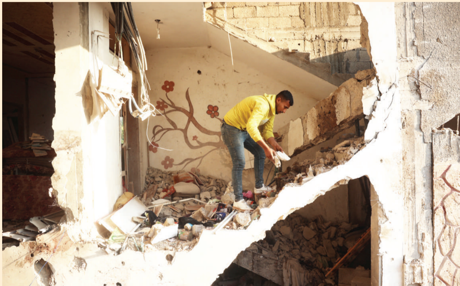
A Palestinian man checks the damage inside a building targeted by an Israeli air strike early on Dec 12, 2024 near the Nuseirat refugee in the central Gaza Strip, amid the continuing conflict between Israel and Hamas. (PHOTO / AFP)
