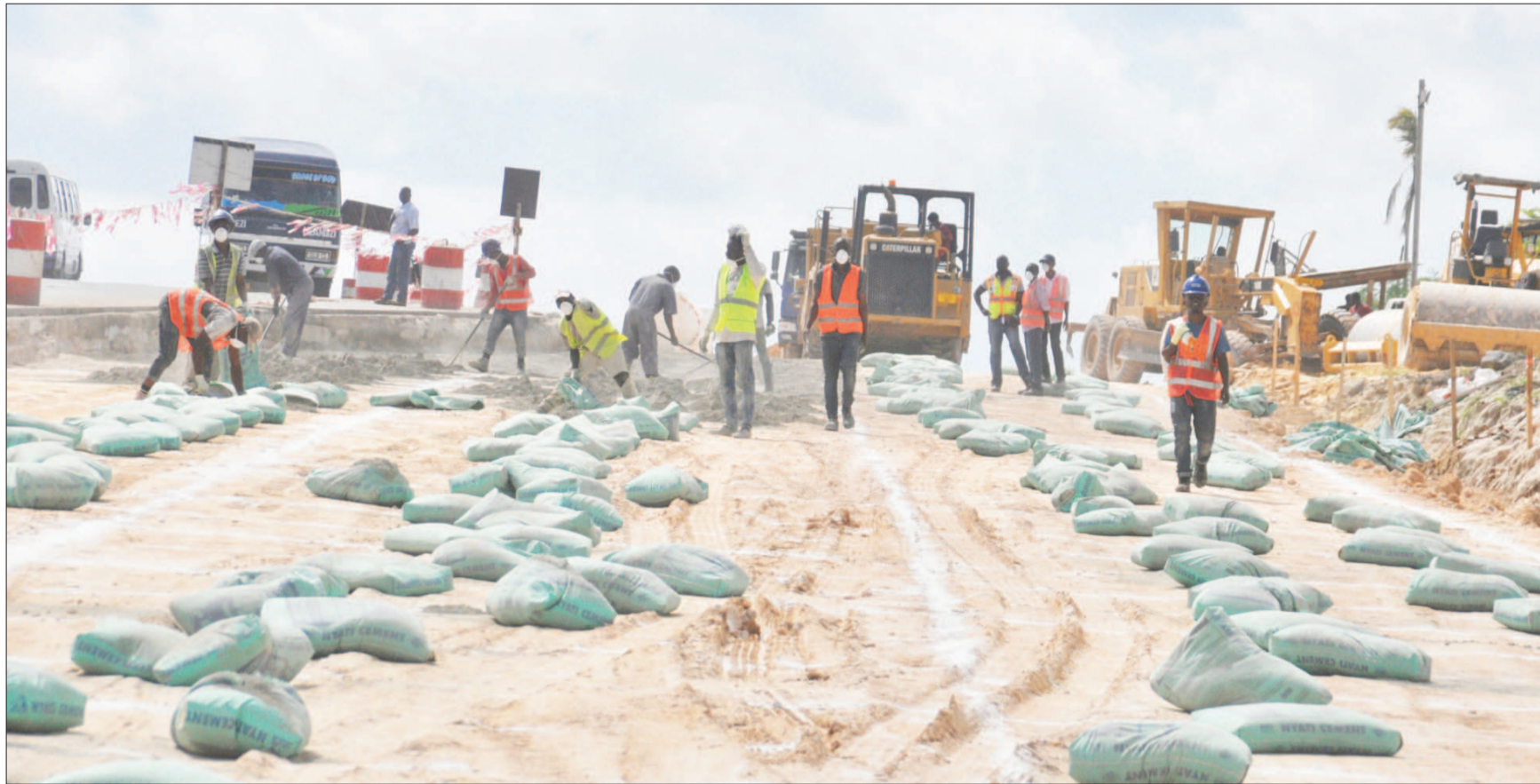
Estim construction company workers at work along the Morogoro Road section of Kimara to Kibaha six lanes dual carriageway phase one including construction of Kibamba, Kiluvya and Mpiji bridges as captured by our photographer at Mbezi Mwisho area in the outskirts of Dar es Salaam yesterday. Photo: John Badi
