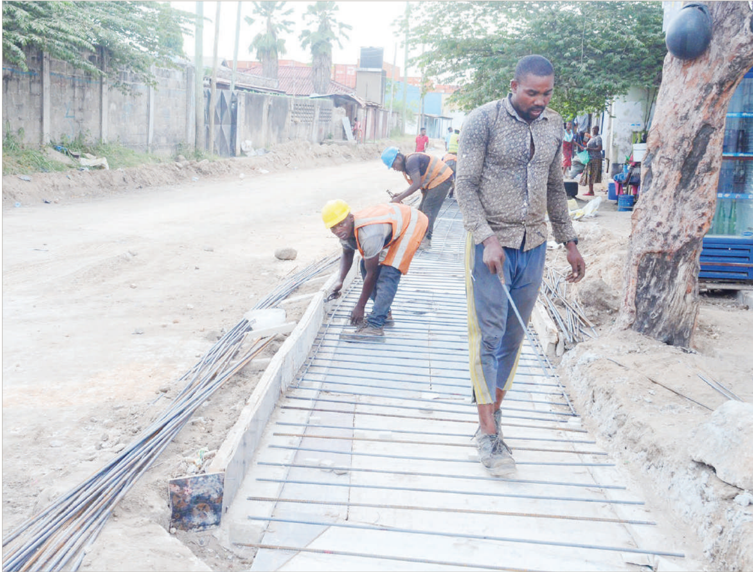
CRJE company sewer construction workers at Kurasini in the outskirts of Dar es Salaam install sewer pipes to transport wastewater out of structures and to a body of water or treatment facility. They dig trenches and insert the pipes, making sure they have correct angle and are connected watertight. Sewer construction workers also construct other elements of sewage infrastructure, such as manholes, and maintain and repair existing systems. Photo: Correspondent Jumanne Juma
