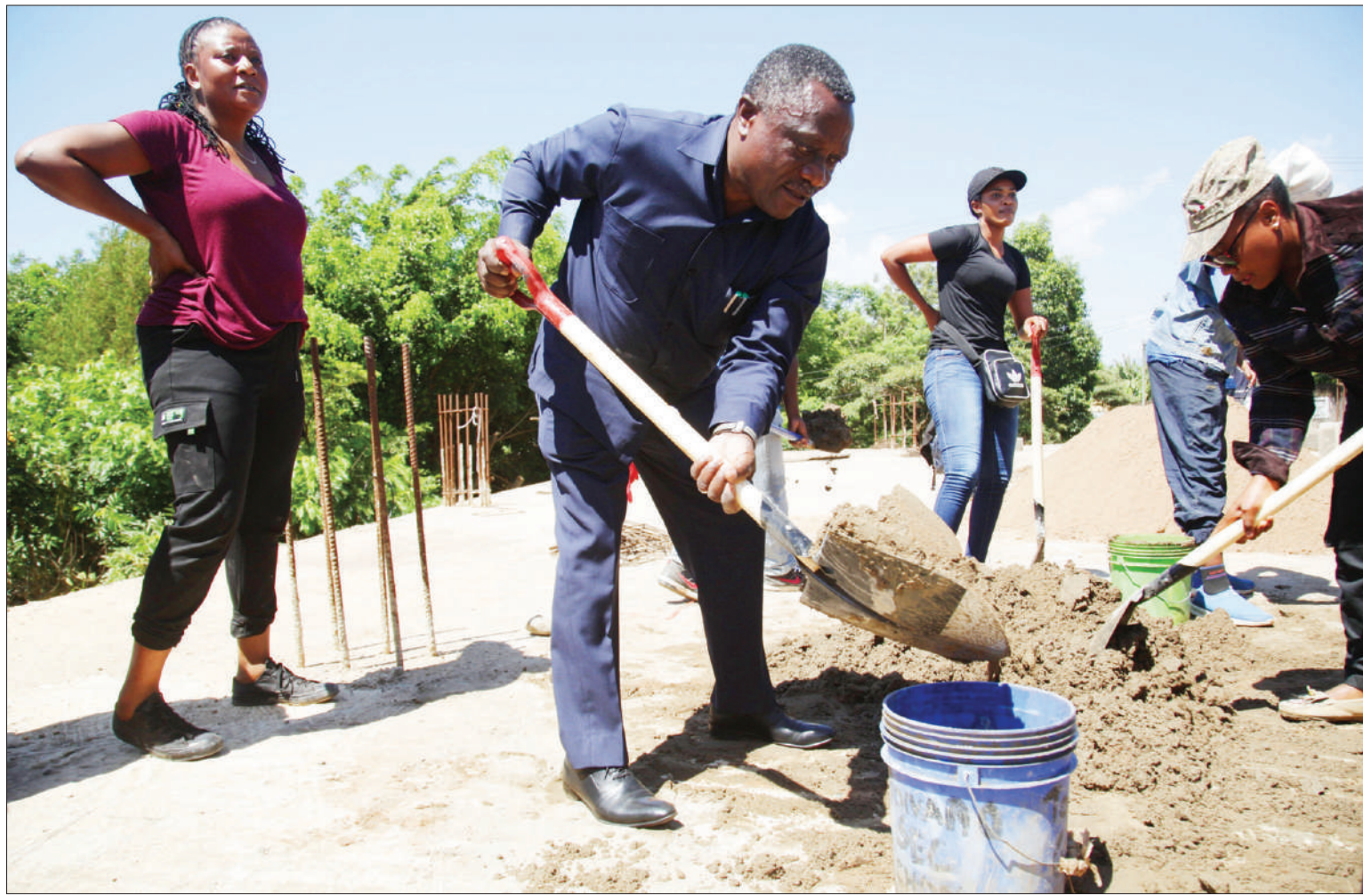
Arusha Regional Commissioner Idd Kimanta participates in construction of classrooms at Elerai secondary school on Tuesday. Photo: Correspondent Getrude Mpezya
