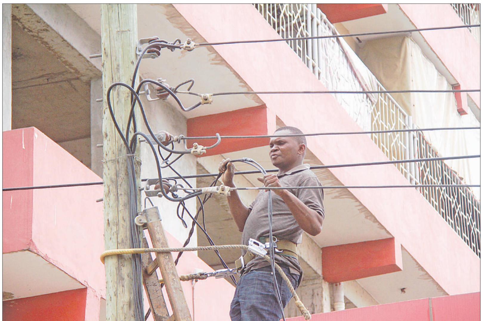
A Tanzania Electric Supply Co. (TANESCO) technician changes wires without protective gear near the Karume Stadium in Dar es Salaam yesterday. Photo: Correspondent Jumanne Juma
