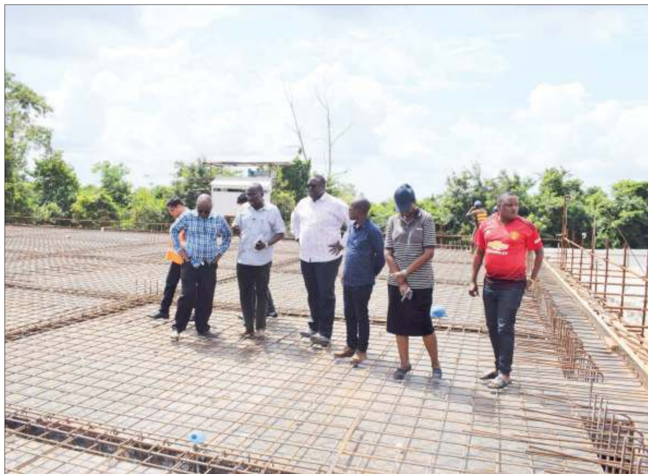
Dar es Salaam Water and Sewage Authority (Dawasa) CEO Cyprian Luhemeja (4th-R) briefs Water ministry permanent secretary Prof Kitila Mkumbo (L, facing camera) at Kisarawe at the weekend on the implementation of a project under which Dawasa will be supplying water to Kisarawe District in Coast Region. Photo: Guardian Correspondent
