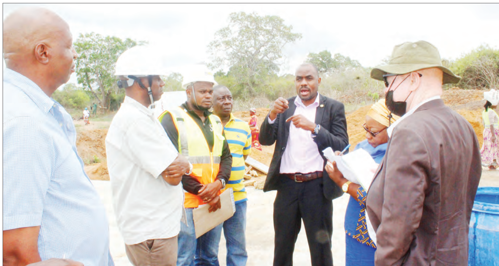
Cashewnut Board of Tanzania acting director general Francis Alfred (C) makes remarks yesterday after visiting the site where a cashewnut factory is undergoing construction in Mkinga District, Tanga Region. Right is Tanga regional cashewnut board manager Ugumba Kilasa. Photo: Correspondent Oscar Kasimiri.
