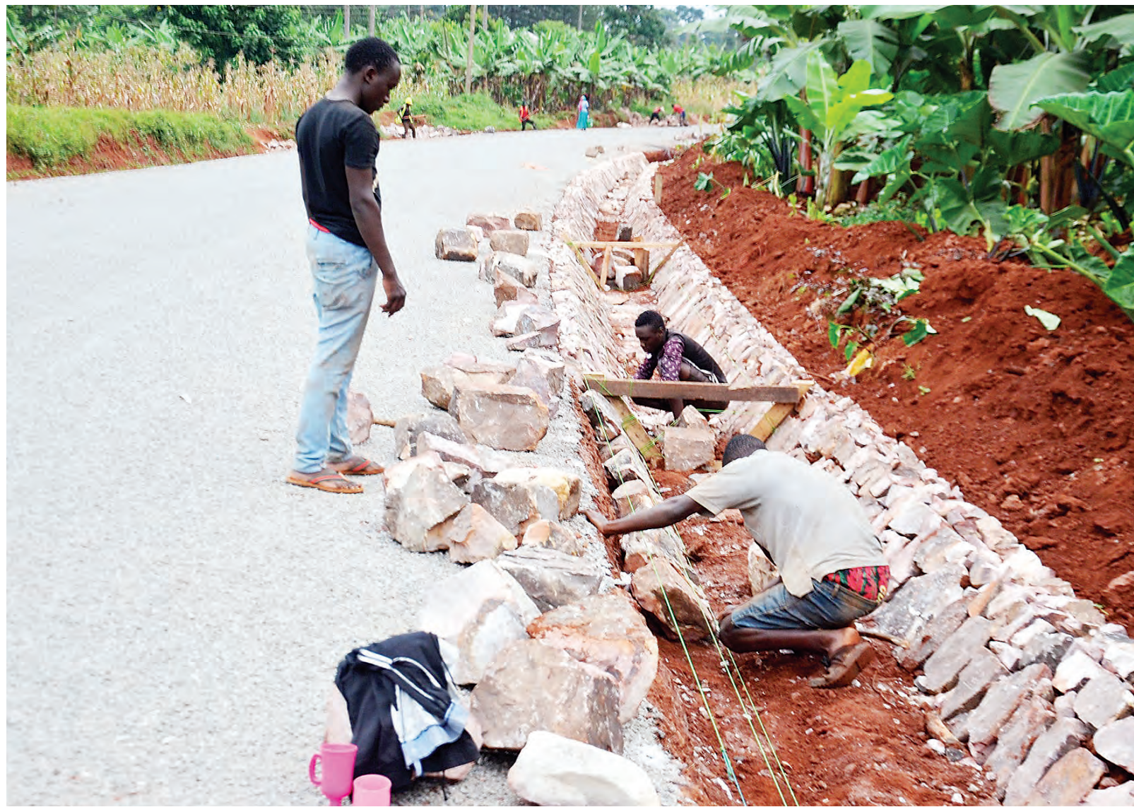
Construction of a storm drain gets well under way beside a newly built road in Mbulu District, Manyara Region, as found earlier this week. Photo: Correspondent Jumanne Juma
