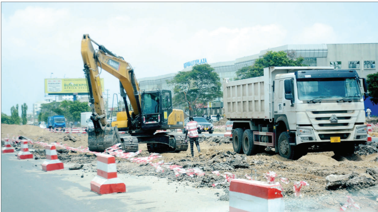
Implementation of Phase III (Gerezani to Gongo la Mboto) of the Dar es Salaam Bus Rapid Transit road construction project well under way, as captured yesterday at the Mtava section of Nyerere Road. Photo: Correspondent Jumanne
