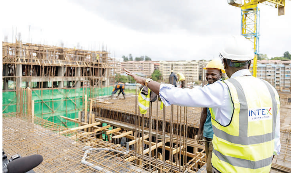
President William Ruto has a word with a construction worker at Kibra, Soweto B Social affordable housing project in Nairobi
