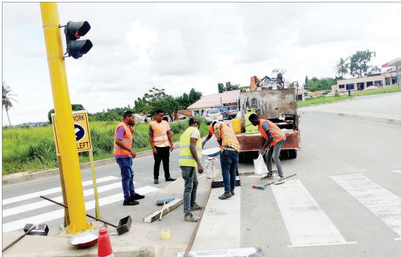
Tanzania Rural and Urban Agency (Tarura) technicians paint a zebra crossing sign at a busy Kimara Stop section of Dar es Salaam's Morogoro Road yesterday. Photo: Correspondent Sabato Kasika
