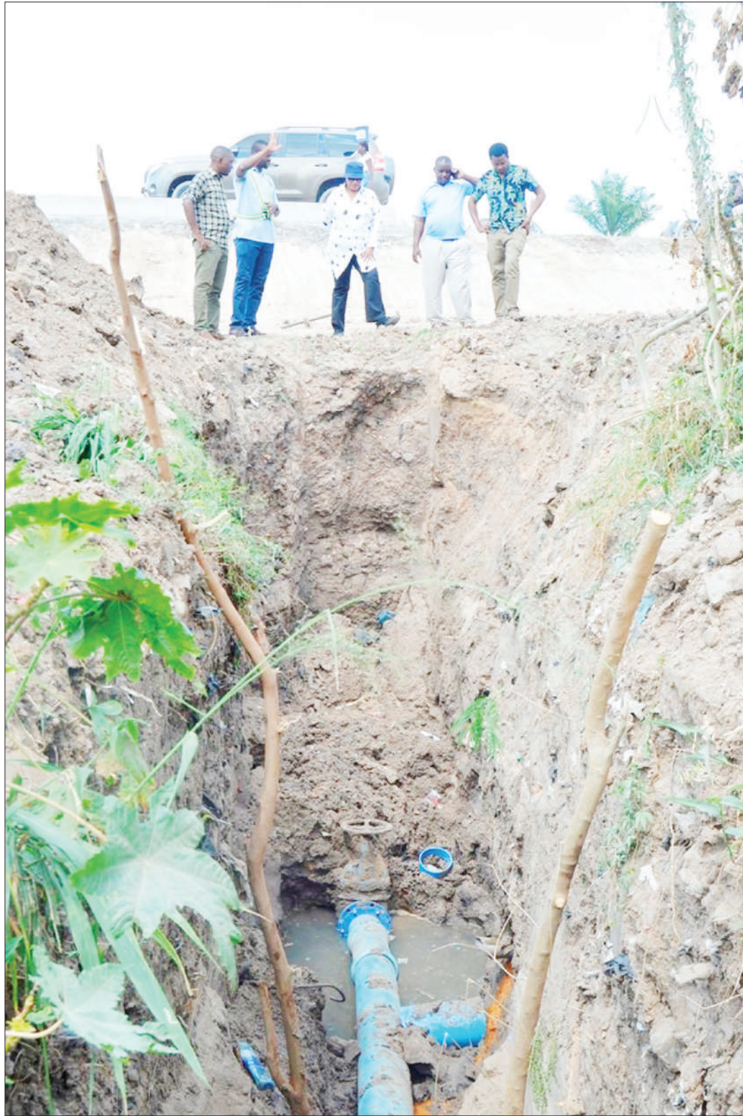
Dar es Salaam Water and Sanitation Authority (DAWASA) community communication director Neli Msuya (C) gets an explanation from Ubungo regional manager Eng Pascal Fumbuka (L) on water pipe construction stretching to about 2.3 kilometers at Mbezi Luis to increase water pressure at Makabe, Uzunguzi, Hekima, Mageti, Kwa Robert, Muhimbili and Matosa Juu. Photo: Guardian Correspondent
