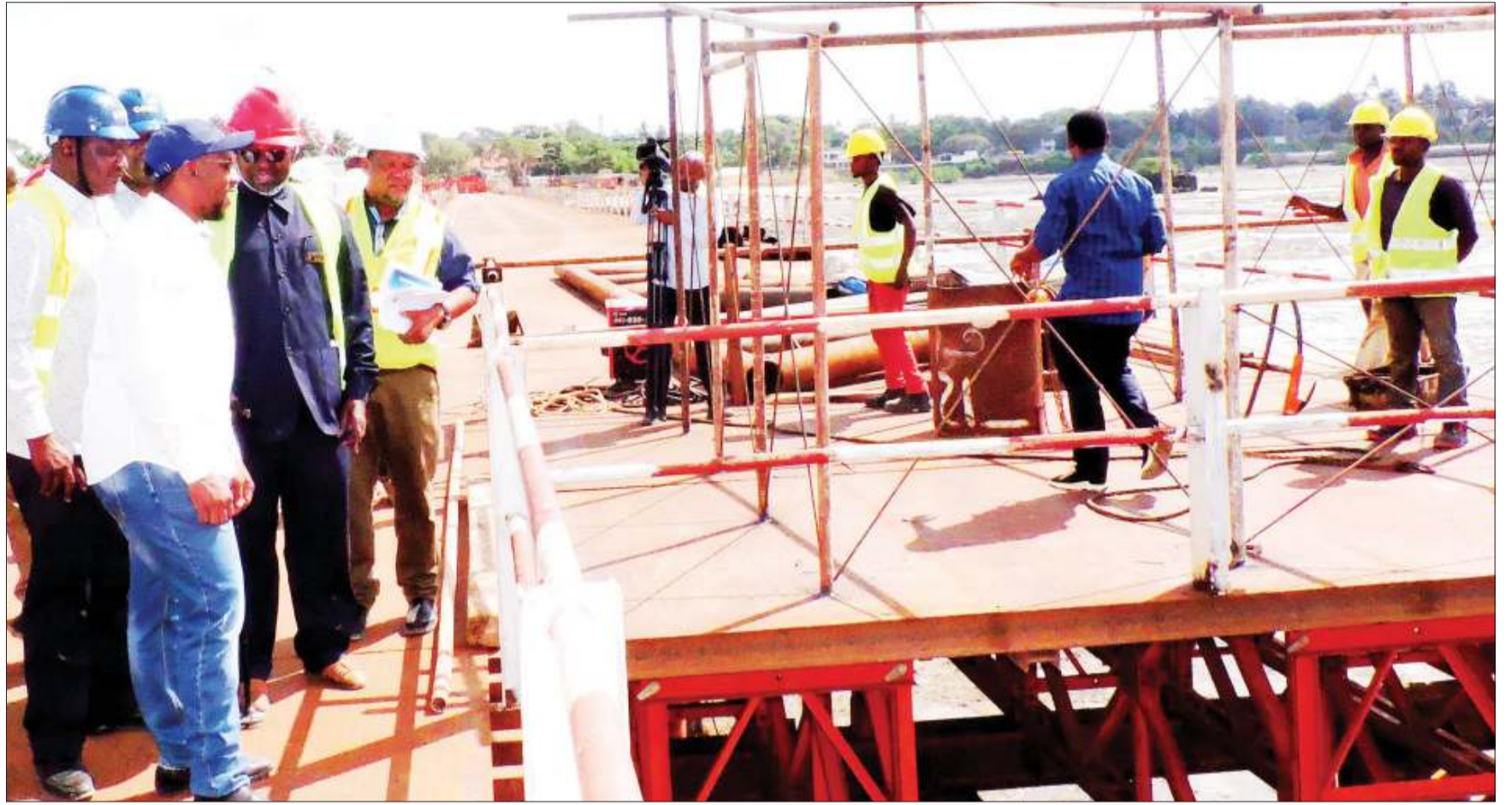
Dar es Salaam Regional Commissioner Paul Makonda (L) inspects temporary construction of a bridge that will link Agha Khan to Coco Beach along the Indian Ocean yesterday. Photo: Correspondent Getrude Mpezya
