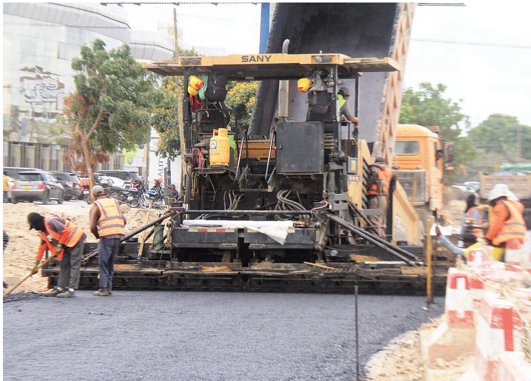
Tarmacking of the Darajani section of the Gerezani to Gongo la Mboto stretch of the Dar es Salaam rapid bus road infrastructure well under way, as found earlier this week. Photo: Correspondent Jumanne Juma
