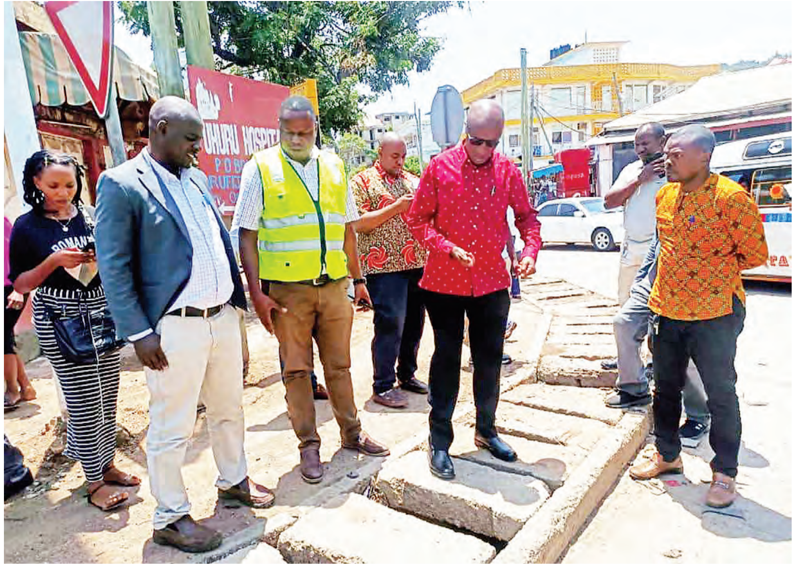
Mwanza regional commissioner Robert Gabriel (in red shirt) directs Tanzania Roads Agency (Tanroads) officials in Mwanza city earlier this week to rehabilitate all drainage systems and other road infrastructure damaged during the relocation of small traders to areas earmarked for them. Photo: Correspondent Rose Jacob
