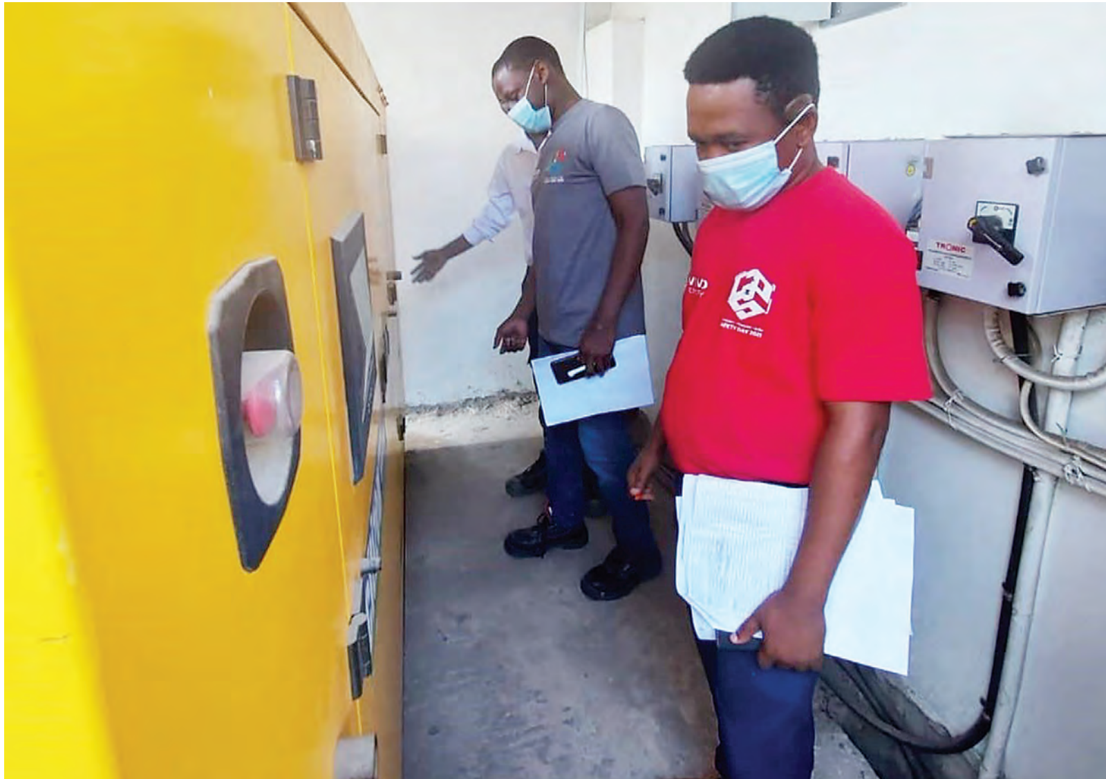
Vivo Energy Tanzania retail engineering manager Joseph Sengavudemu (L) and territory manager Mohamed Abdullah check the state of the firm's generators at a retail sales site during its annual Safety Day held in Dar es Salaam earlier this week, all in line with health, safety, security, environmental and quality considerations. Photo: Guardian Correspondent
