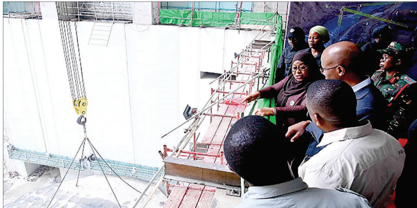
President Samia Suluhu Hassan (C) listens to Energy minister January Makamba and TANESCO managing director Maharage Chande after launching water diversion and start water filling at the Julius Nyerere hydro power plant along Rufiji River yesterday. Photo: State House
