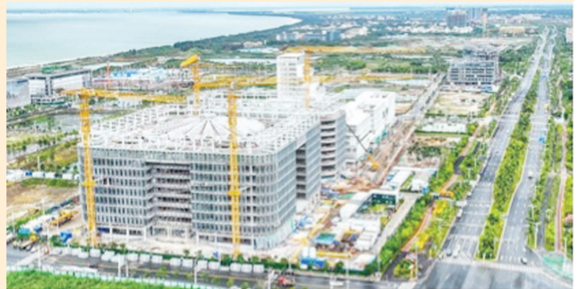
The headquarters of the Bank of Hainan in Haikou, south China's Hainan province is under construction, November 2022. (Photo by Zhang Mao/People's Daily Online)
