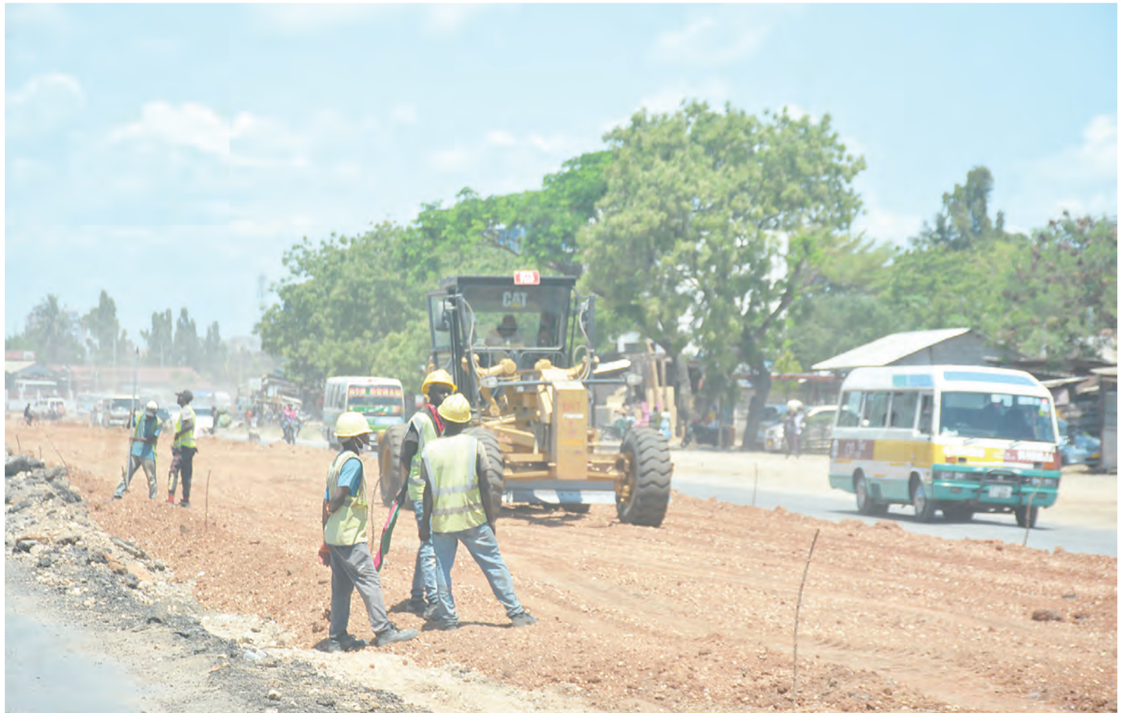
Implementation of Dar es Salaam's Bus Rapid Transit road construction project in progress along the Magomeni stretch of Kawawa Road yesterday. Photo: Correspondent Jumanne Juma
