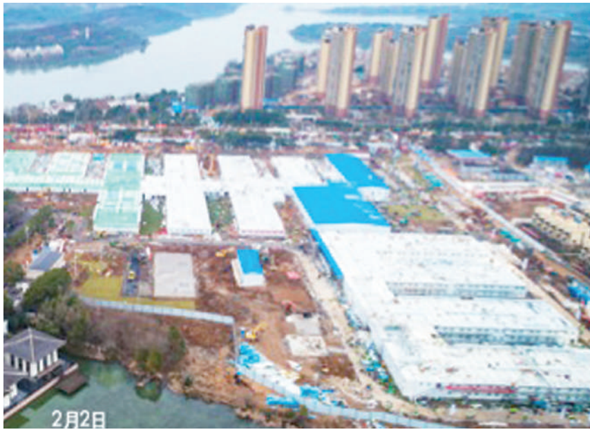
It takes only 10 days to complete the construction of the Huoshenshan Hospital, a makeshift hospital in Wuhan to battle against the novel coronavirus outbreak. (Xinhua)
