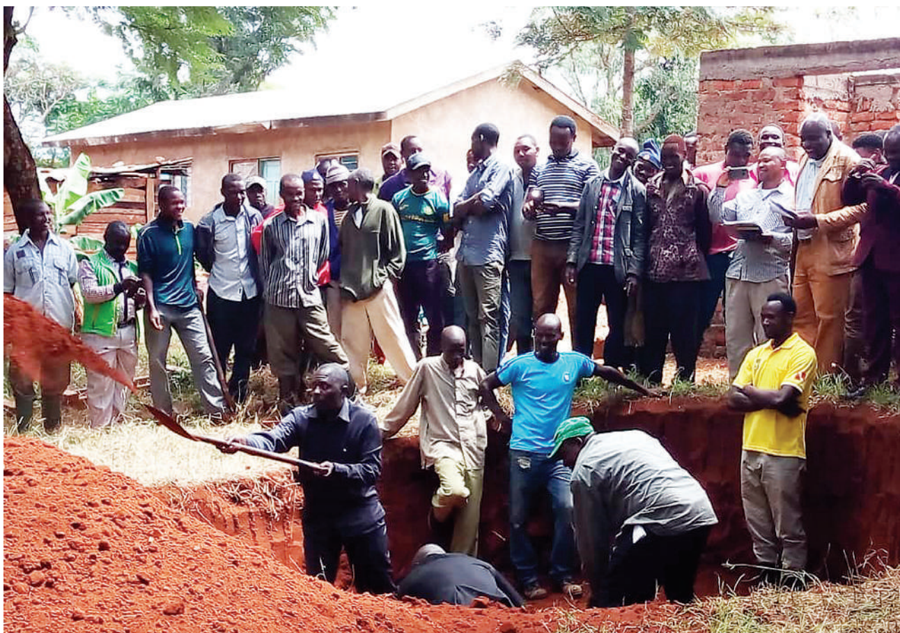
Siha district commissioner Onesmo Buswelu (L, with spade) pictured yesterday participating preparatory work expected to lead to the construction of improved pit latrines for teachers at Namwai School. Photo: Godfrey Mushi
