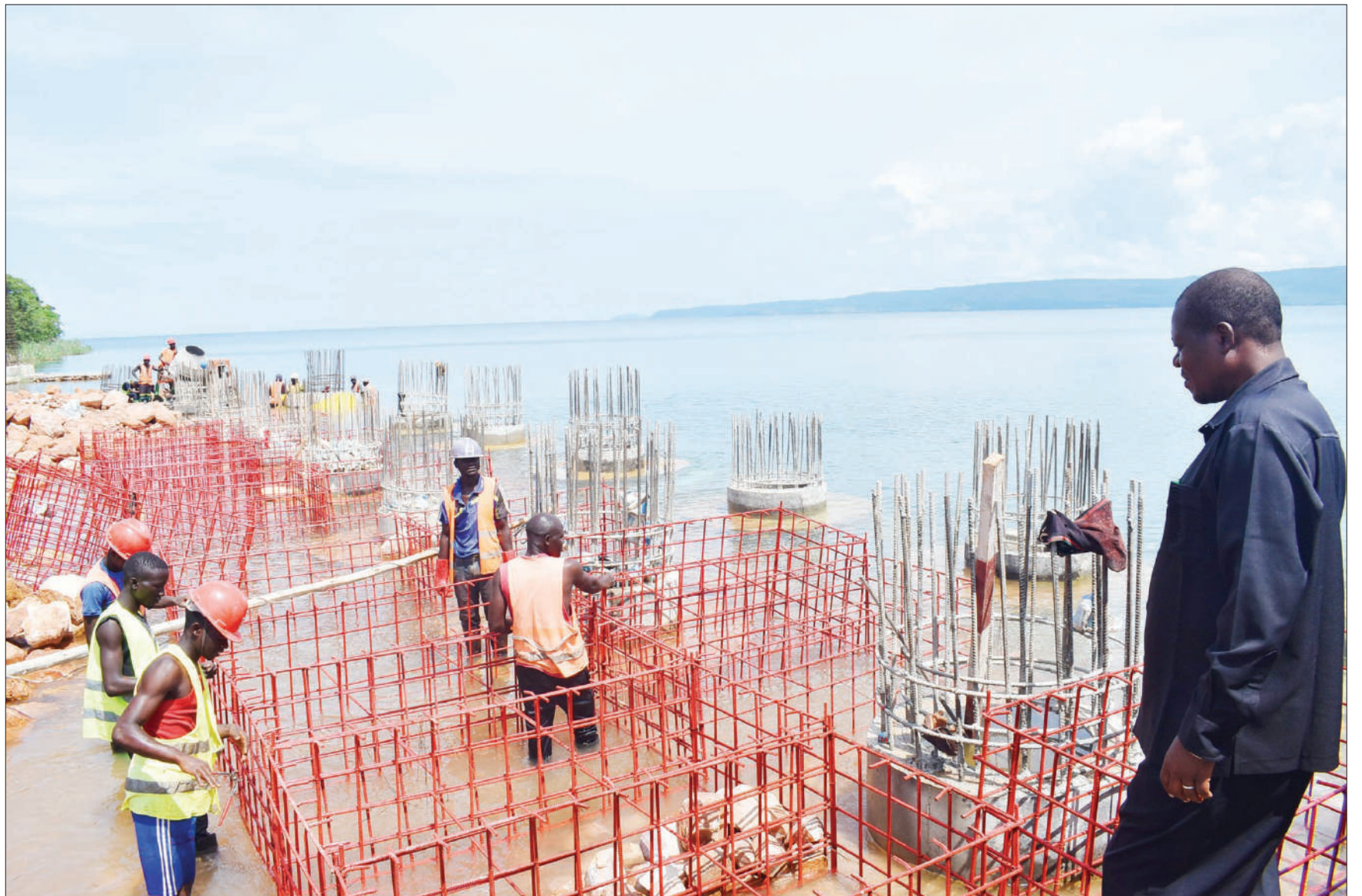
Rukwa regional commissioner Joachim Wangabo (R) pictured yesterday inspecting progress in the expansion of Kasanga harbour dock on the Tanzanian side of Lake Tanganyika, work meant to enable two ships to anchor at the facility at a go. Photo: Guardian Correspondent
