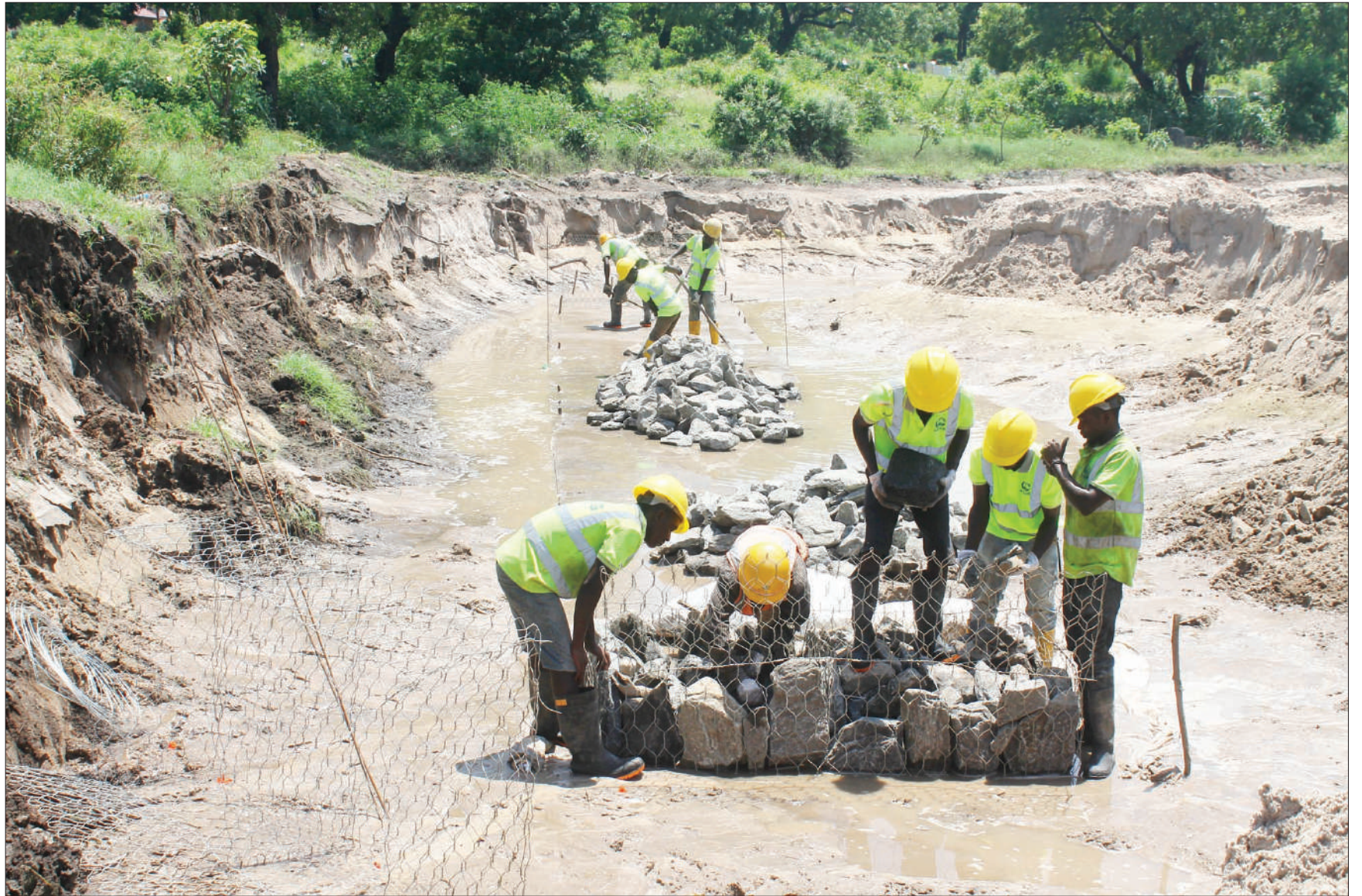
China Railway Seventh Group workers lay the groundwork for the construction of a sewage system at Chang'ombe in Dar es Salaam yesterday. Photo: Correspondent Jumaine Juma
