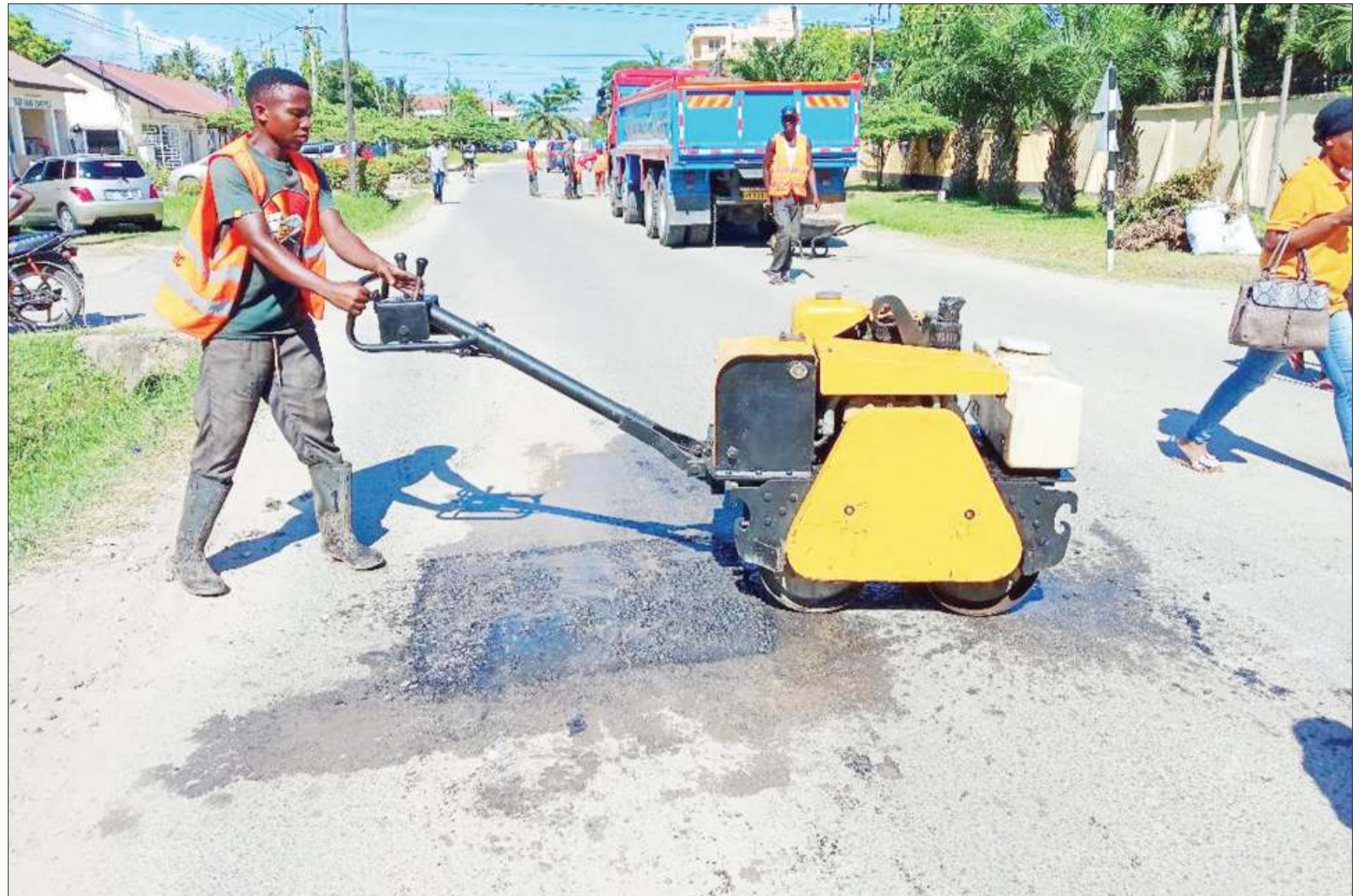
Repair of a road near Dar es Salaam's Hubert Kairuki Memorial Hospital under way yesterday. Photo: Correspondent Joseph Mwendapole
