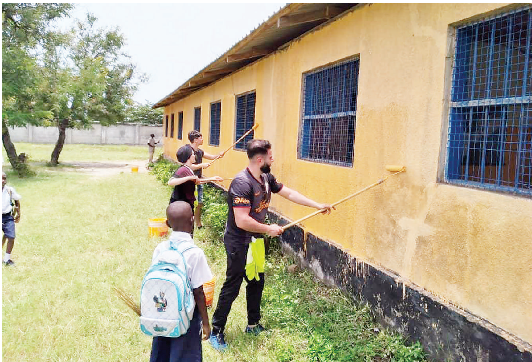
Kawe B primary school student look at the volunteers from Time To Help Netherlands when they were decorating his school with new paint. The school was in bad condition before the renovation. (Photo: Guardian Correspondent)
