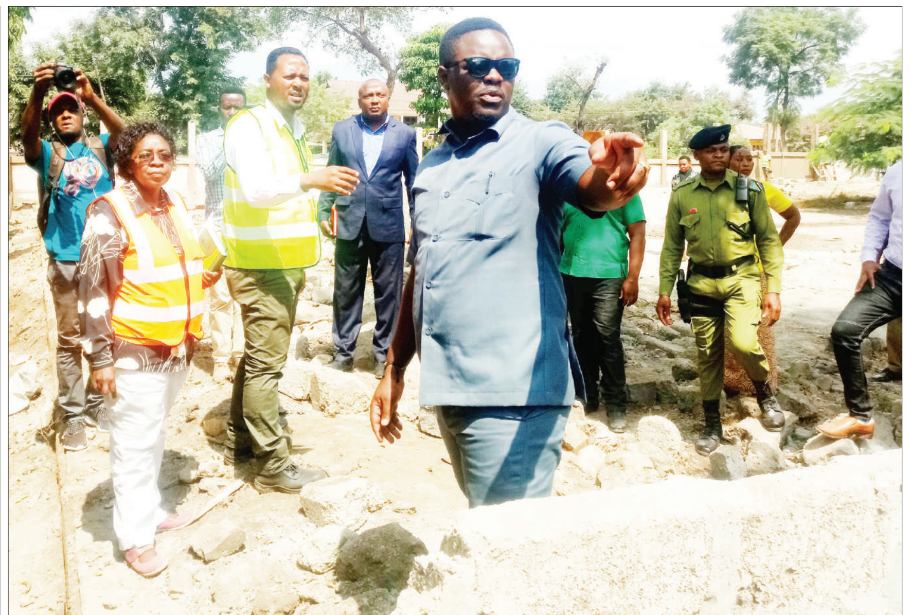
Hai district commissioner Lengai ole Sabaya (in dark glasses) visits the site of a 50m/- Tanzania Electric Supply Company (Tanesco) project where construction is in progress, as captured yesterday. Photo: Godfrey Mushi
