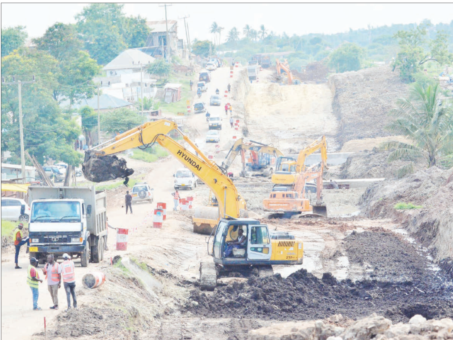
Rehabilitation of a service road under way at Mbezi Mwisho in Dar es Salaam yesterday to facilitate the ongoing expansion of expansion of part of Morogoro Road. Photo: Correspondent Miraji Msala
